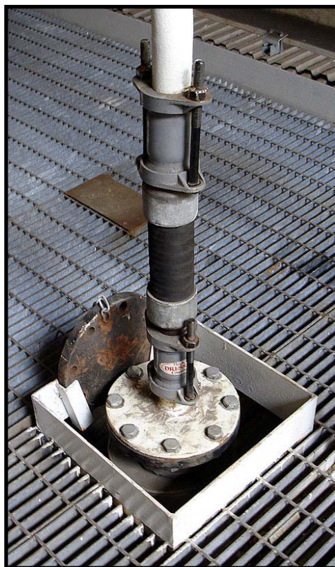
Duct Injection Port
