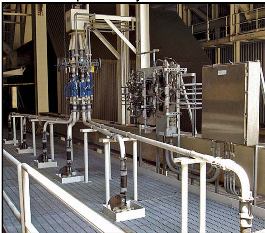
Splitter to Injection Ports
