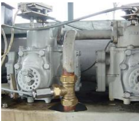
Figure 27 Typical installation of temperature sensor
