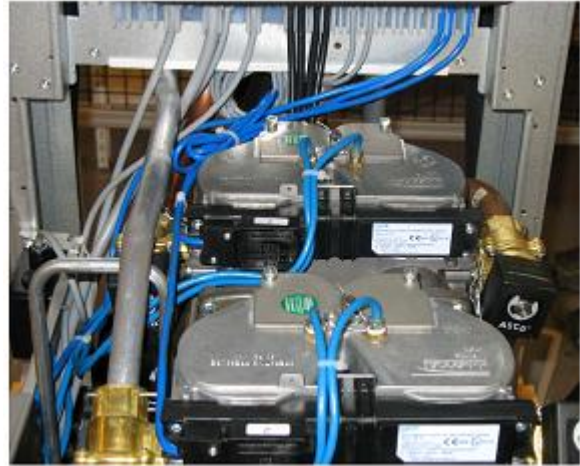
Figure 34 Probes mounted in dome cover
