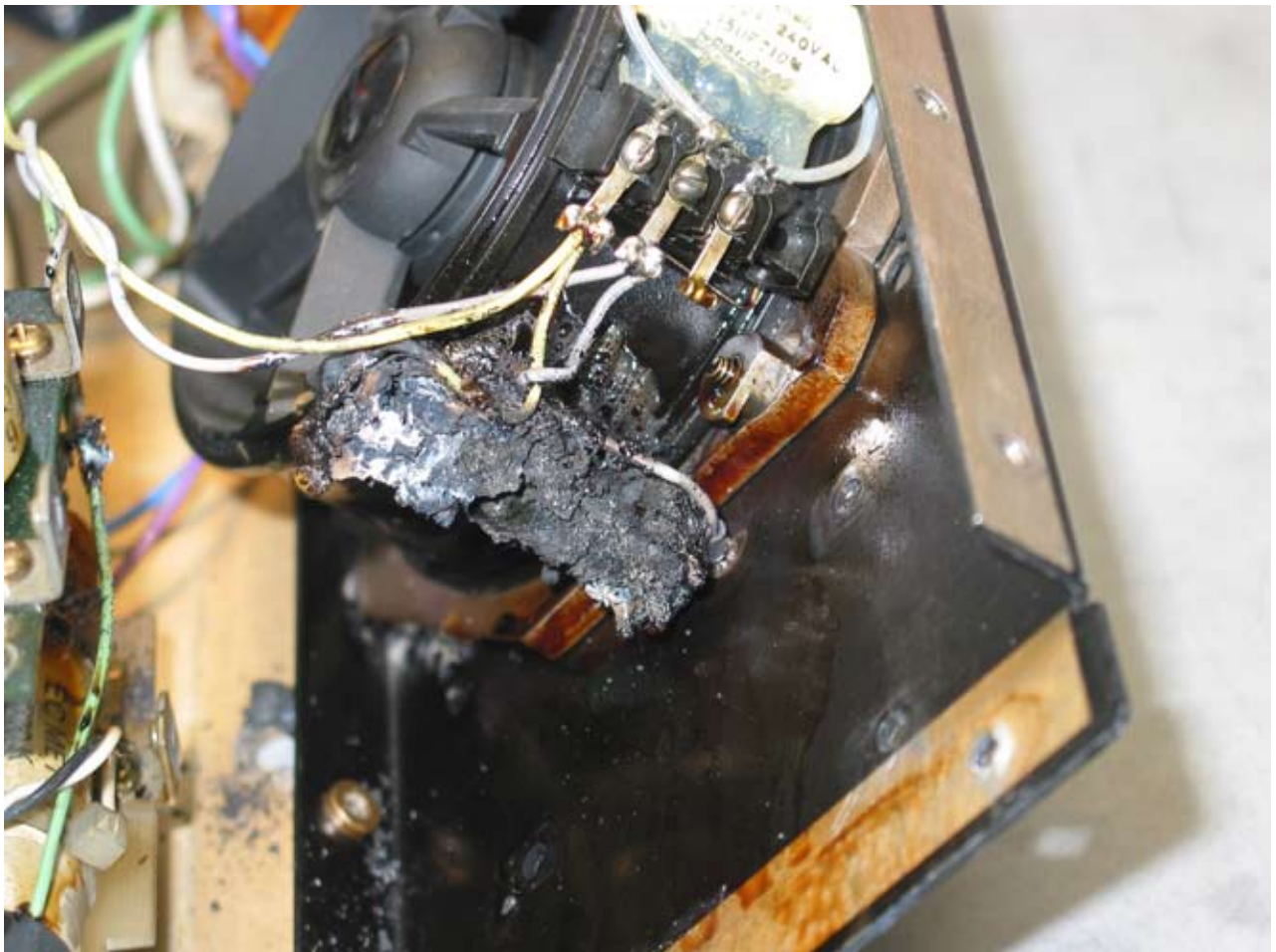
Figure 1 Burnt out capacitor
