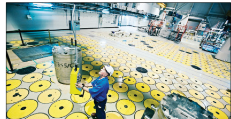
Inside the Vitrified High Level Waste Store
