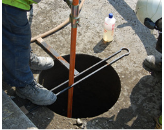
Figure 12 - Reinstating unbound material in layers, and checking compaction with a peizo sensor and a compaction monitor
