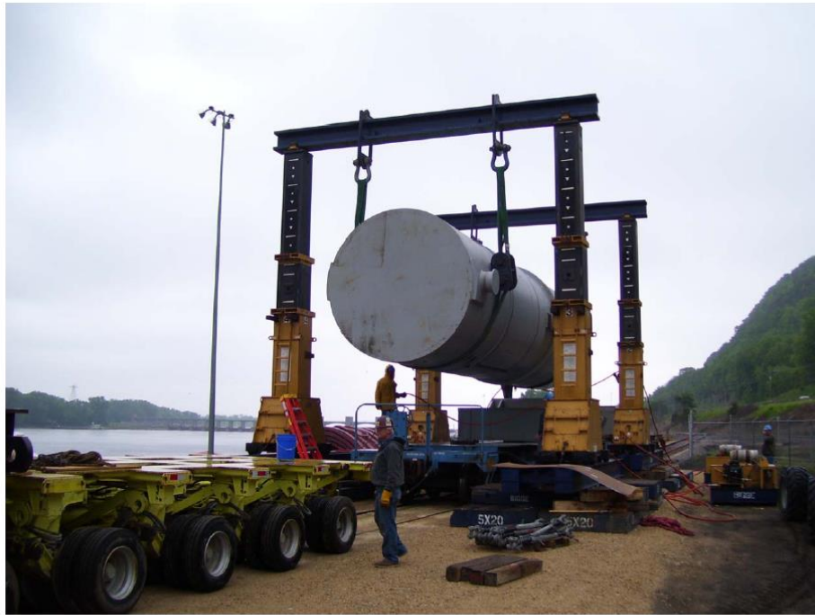
Transfer of RPV transportation package from the heavy hauler to the rail cars
