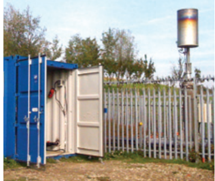
Pilot scale flue gas capture plant at North Farm landfill site, Tunbridge Wells, Kent
