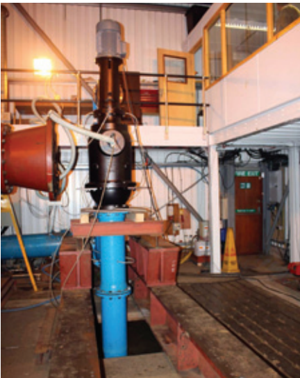
Saxtal aerator being tested
