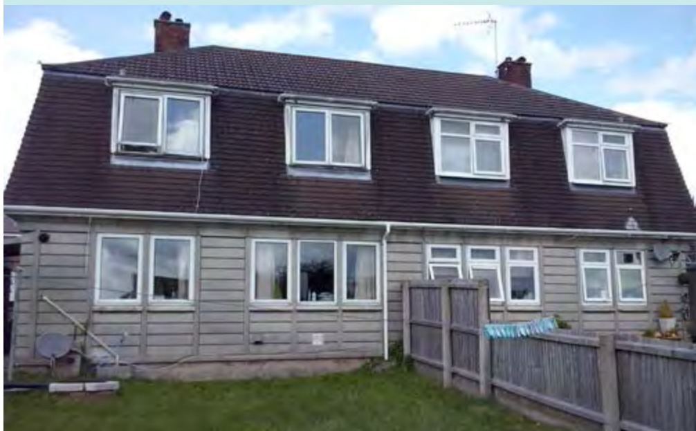
A similar unrefurbished property on the same estate
