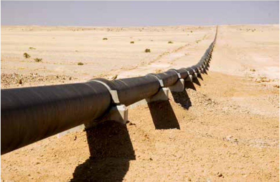
A water pipeline to Paladin Energy's Langer Heinrich Uranium Mine
