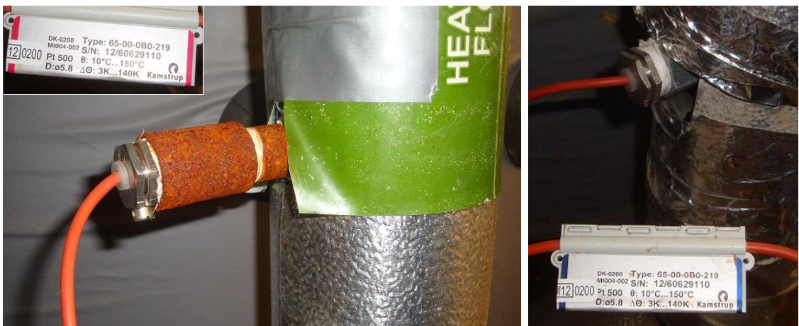
Figure 63 – A made-up fitting and a correct fitting used on the same heat meter.
