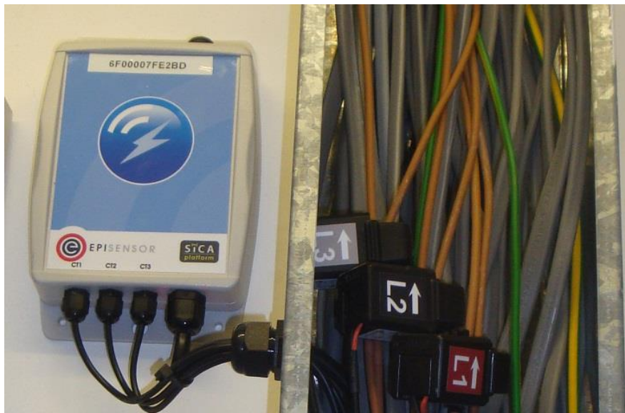
Figure B 7 – ZEM-61 3-phase electricity monitor with current transformers installed in cable trunking.
