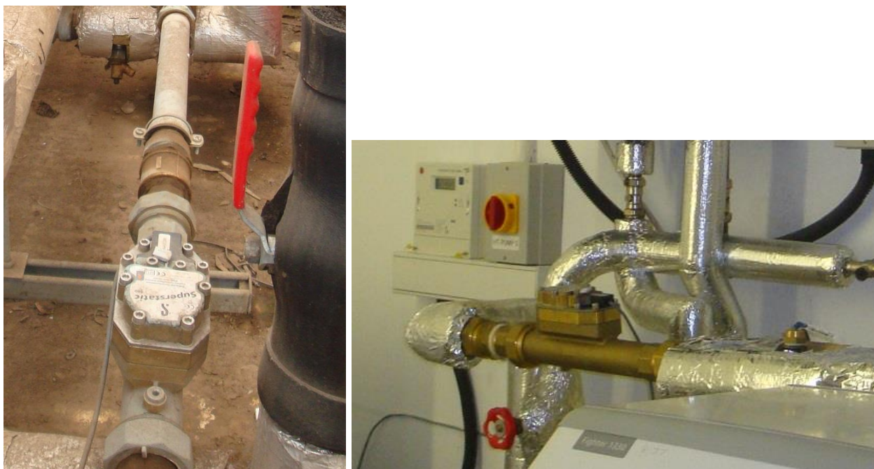
Figure 68 – Incorrectly mounted vortex flow meters
