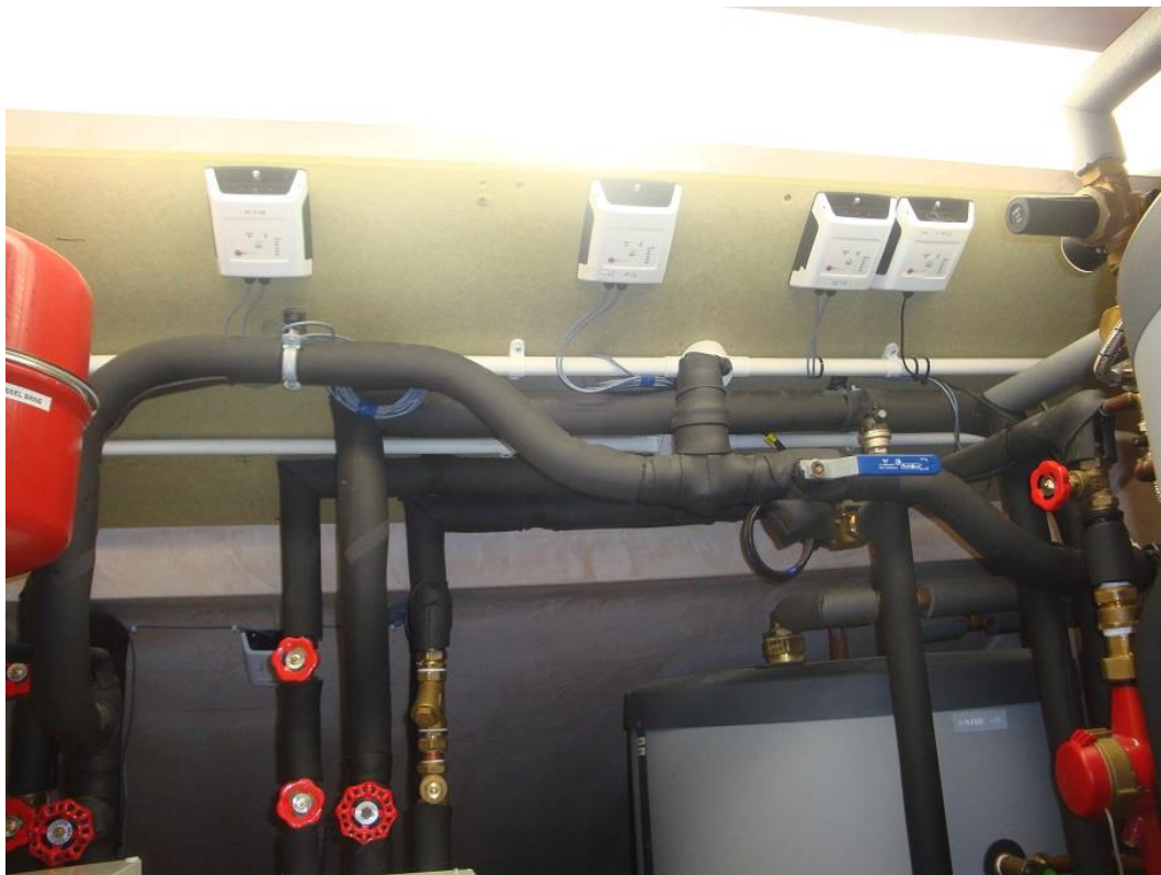
Figure B 11 – TES-32 temperature sensors mounted on the ceiling of a plant room.
