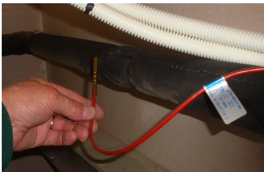
Figure 65 – Loose temperature sensors on the wrong pipes
