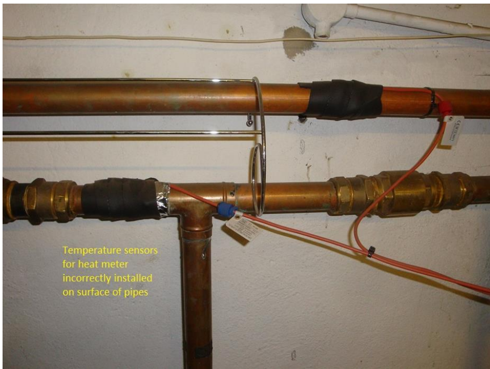
Figure 64 – Strapped on temperature sensors
