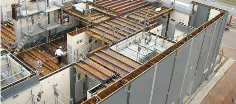
Steele concrete steel (SCS) construction of a module in a nuclear power plant.
