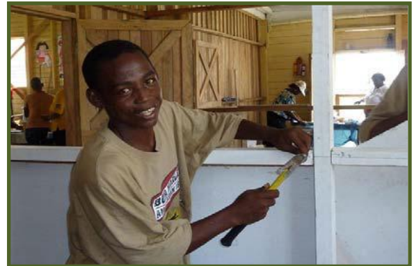
A trainee carpenter helps refurbish the All Saints community centre in New Amsterdam, Guyana, along with other women workers as part of a vocational training course funded by DFID through UNDP's Enhancing Public Trust, Security and Inclusion programme
