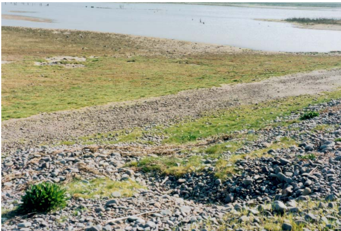
Figure 10 Seepage “cans” on the backslope or landward face of the barrier near to the War Memorial close to profile E10. These features are characteristic of active gravel barriers and are formed by seepage of sea water through the barrier during periods of high water level in the bay. Note that seepage pressure is sufficient to displace material resulting in deposition of debris fans a short distance landward. A strand line of flotsam indicates a recent maximum extreme water level of 6.3mO.D. in the lagoon, possibly during the event that formed the can. This level is almost certainly lower than the corresponding Bay extreme level so the hydrostatic gradient thus produced may explain the high seepage pressures generated. Note that flooding of the lagoon partly equalises these pressure gradients reducing seepage and maintaining barrier integrity. Seepage is also inhibited by poorly sorted sediments, wider barriers and vegetation.
