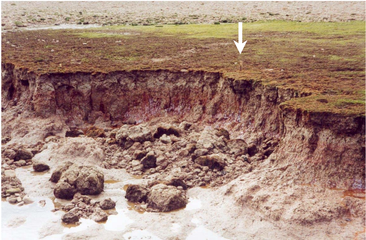
Figure 31. Marker stake located at the margin of the breach channel. Note the cliff fall immediately in front of the stake. The stakes were moved back from the cliff edge as recession progressed.
