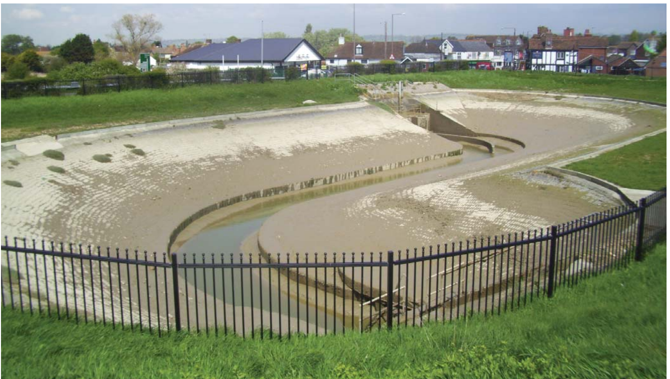
↑ Outfall at Dymchurch, Romney and Walland Marshes.
