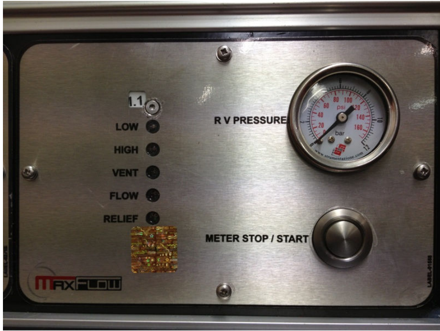
Figure10 Typical view of special gas extractor control unit (electronic) showing hologram seal on Maxflow controller
