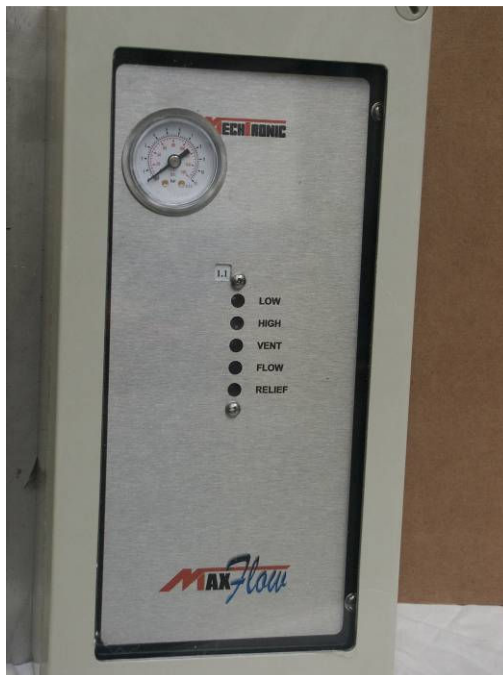
Figure 11 Typical view of special gas extractor control unit (mechanical)
