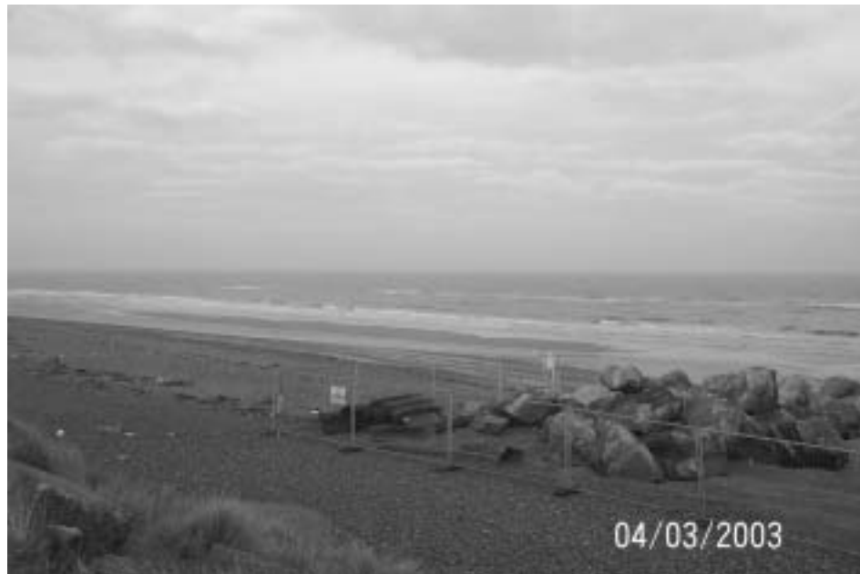
Figure 6.4. Fencing around an active construction work area. Security guards were also used (courtesy Van Oord)
