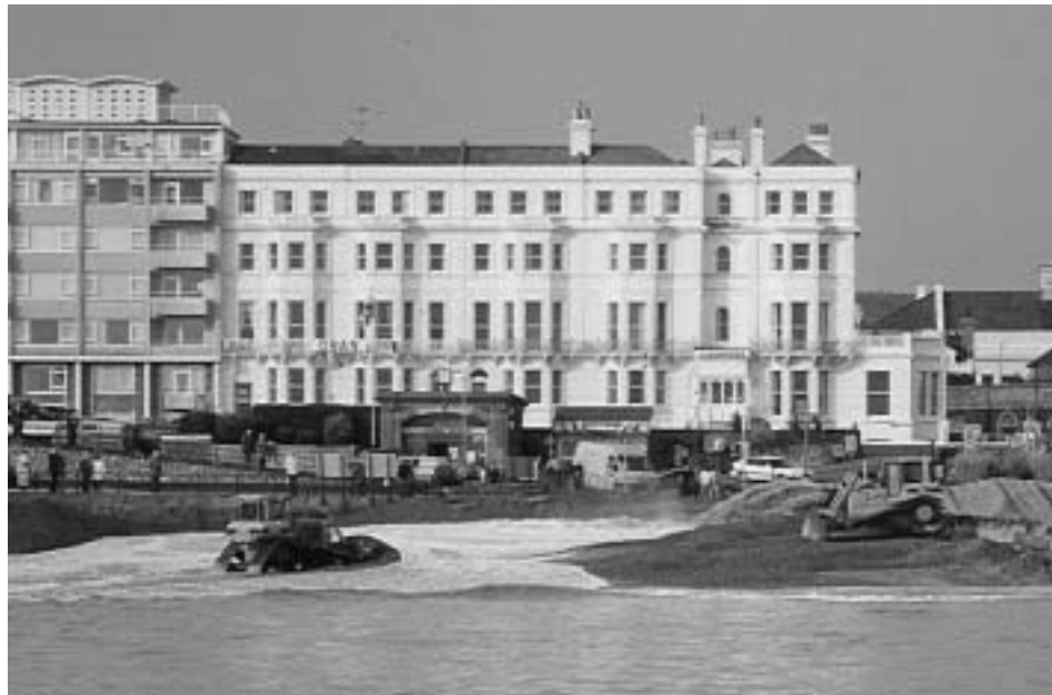
Figure 6.3. Note the problems of working in close proximity to the public (courtesy Van Oord)
