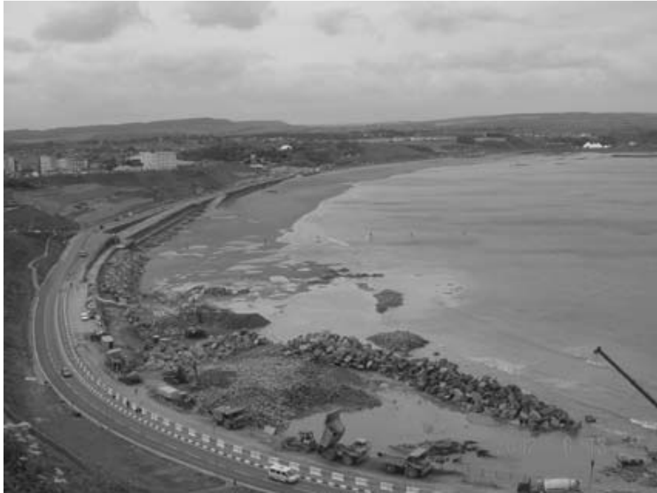
Figure 5.1. Use of conventional land-based equipment in sea defence work (courtesy Edmund Nuttall)
