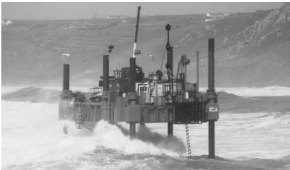
Figure 4.3. Jack-up platform working in exposed wave conditions in Sennen Cove (courtesy Seacore)
