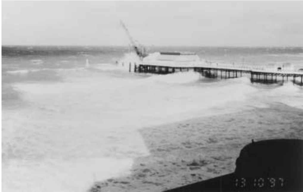
Figure 5.5. Cromer Lifeboat Station under construction, illustrates problem of sea breaking on formwork support under a NW Force 8 (courtesy May Gurney)
