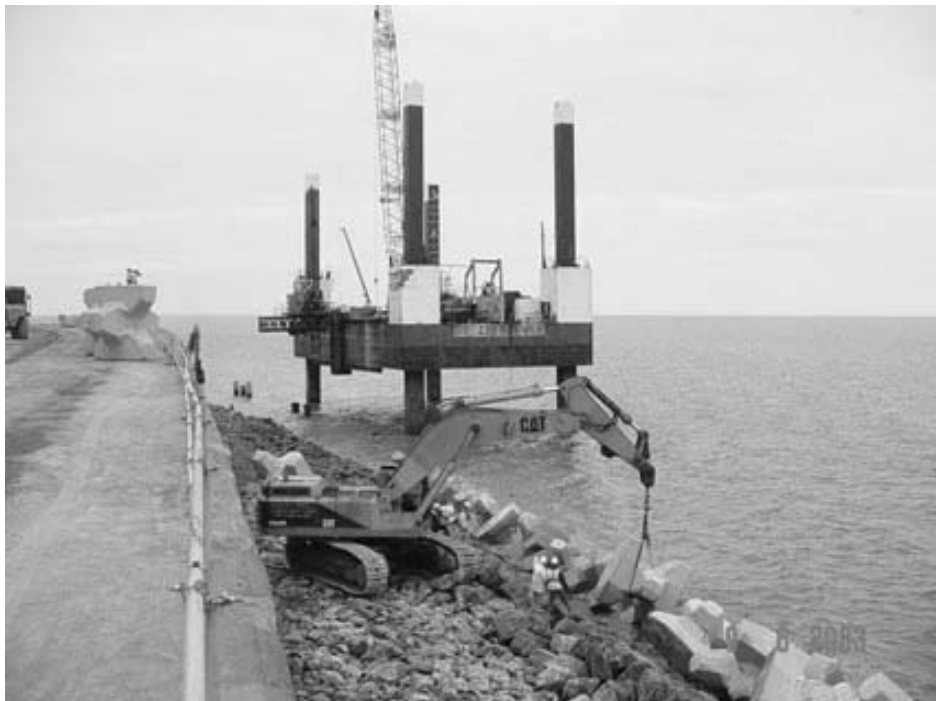
Figure 5.2. Land-based equipment used for placing armour units with jack-up barge behind (Note limited access and working area) (courtesy Edmund Nuttall)
