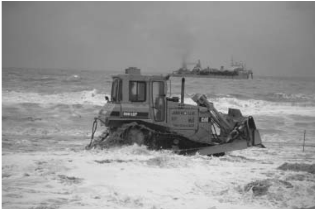
Figure 5.4. Example of earth-moving plant working in a dynamic environment (courtesy Van Oord)
