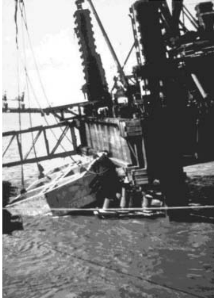
Figure 4.7. Jack-up platform collapsing. Investigation concluded that the jack-up leg possibly penetrated historical borehole (courtesy Tony Edmundson)
