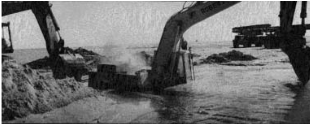
Figure 4.6. Excavator on a rising tide in an outfall trench. Problem caused by bank collapse. Despite appearances the machine was recovered before inundation by the rising tide (courtesy May Gurney)
