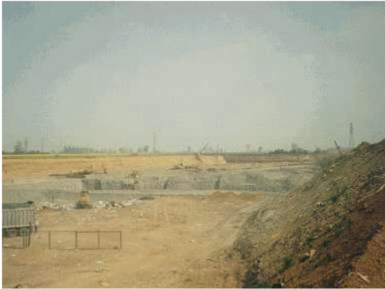
Figure F6.1 Overview of Cell Construction and Waste Infill Operations at the Site
