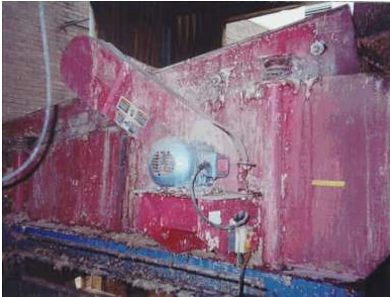
Figure F4.3 The Vibrating Screens Installed at the Factory
