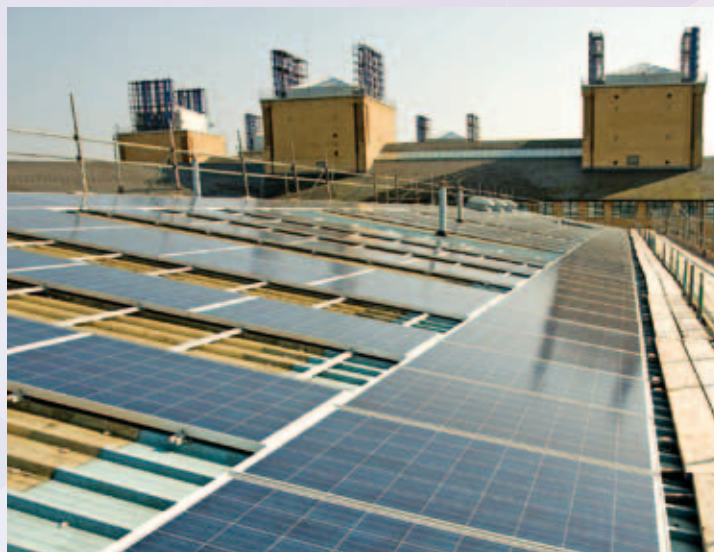
Solar panels on the roof of the Southampton Oceanography Centre.
