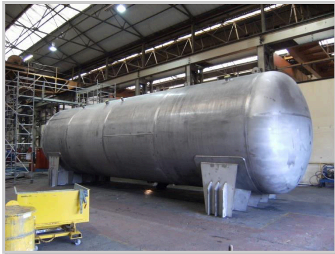
Sludge Storage Vessel
