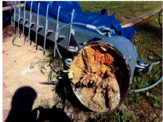
Failed timber post
