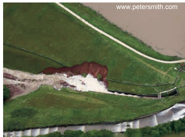
Damage to the masonry channel and dam
