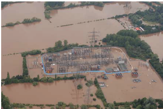
Walham sub-station surrounded by floods
