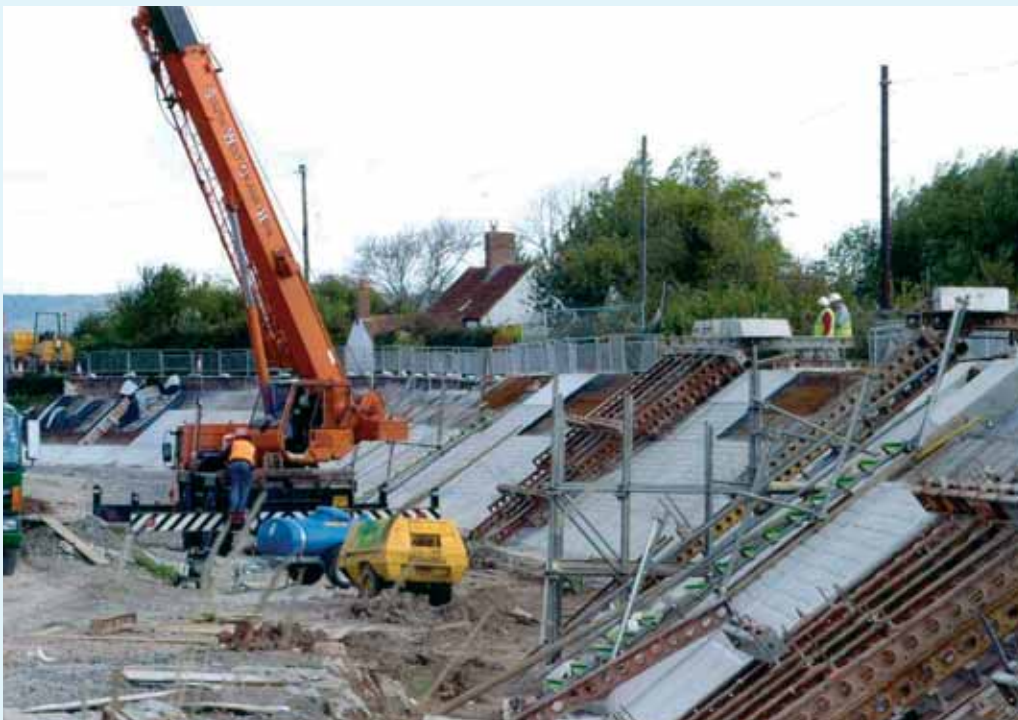
↑ Strengthening the historic Baltmoor Wall on the River Tone, one of many flood defences we manage in the catchment
