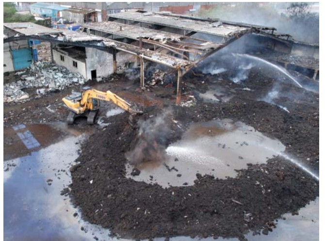
Figure 3: Digger-created lagoon for cooling and extinguishing – Fforestfach tyre fire, Swansea (courtesy of Dr Jorg Hoffmann, Public Health Wales)
