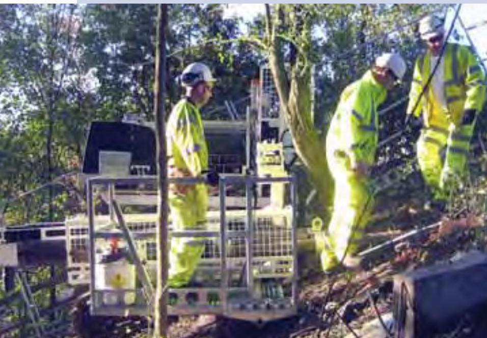
Electro-osmosis: a small crawling rig installs anodes and cathodes into the ground
