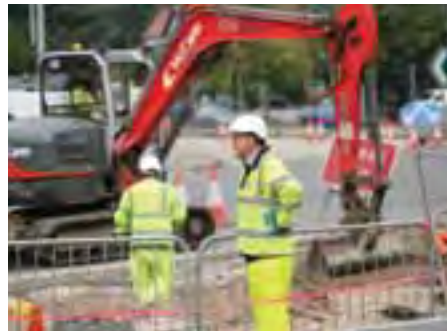
A52 Bramcote to Queens Medical Centre Works include signalling and laying down new road surfaces. Pedestrian crossings and existing signalled junctions along the A52 were upgraded and the carriageway widened at junctions to improve capacity.
