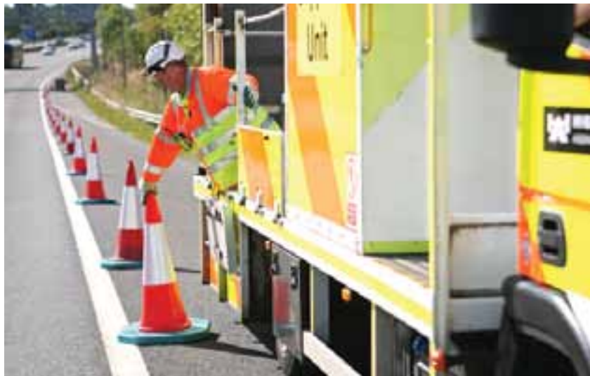
Incident Support Unit laying out cones from the safety of the support vehicle in preparation for roadworks
