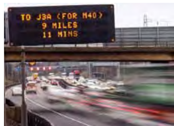
Variable message sign (VMS)
