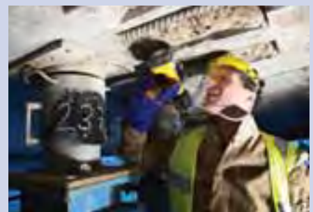
Inspecting the damage at Deans Brook viaduct
