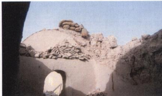
Fig 1-7 Collapsed Roof of Accommodation Building
