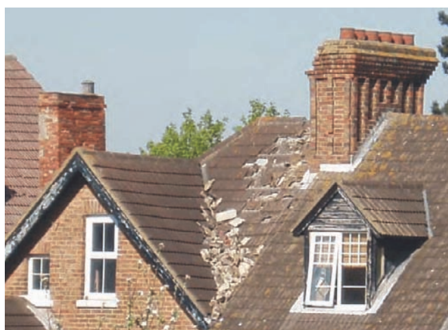
Figure 4: Chimney and roof damage in Folkestone (S. Sargeant ©NERC 2007).
