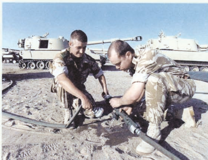
Kuwait, October 1994 – Royal Engineers (attached to 45 Commando Royal Marines) connecting a water supply
