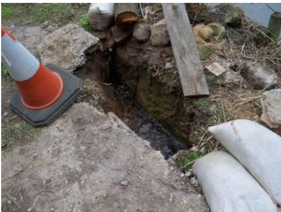
Photograph showing a hole in the embankment with water flowing through
