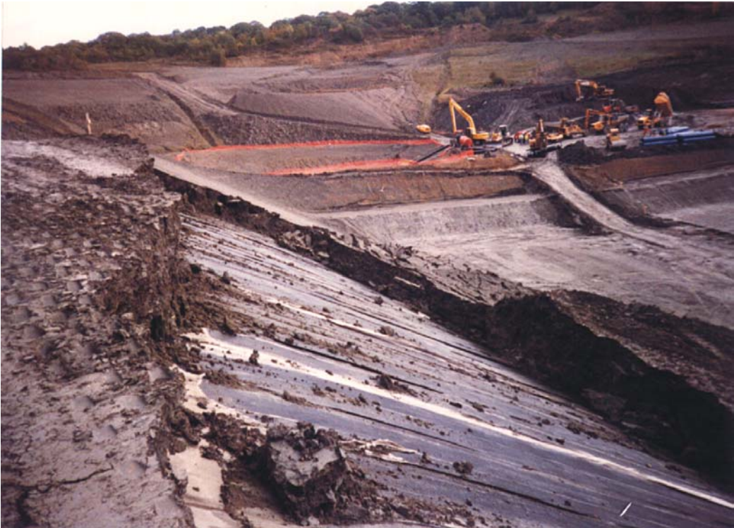
Figure 4.3 Post failure conditions at the site of Case Study No 2
