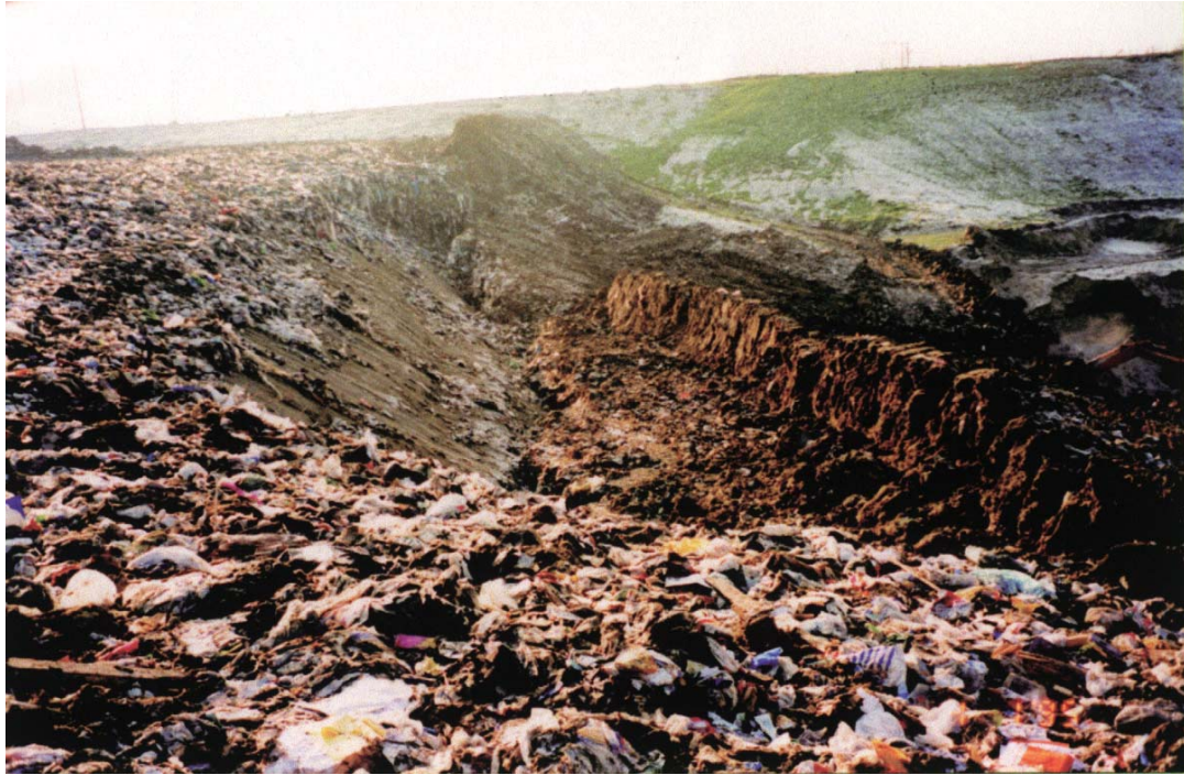
Figure 4.9 General view of the waste slope failure showing the soil covered relic slope
