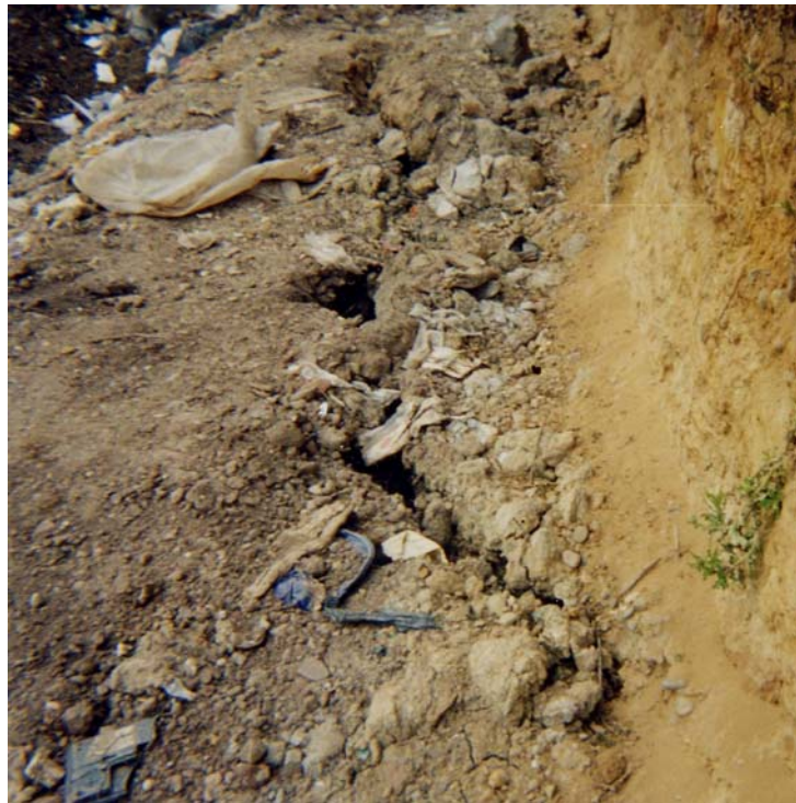
Figure 4.5 View of the tension crack at the rear of the liner caused by toppling failure
