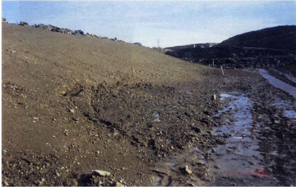
Figure 4.6 View of slumped areas of softened compacted clay liner
