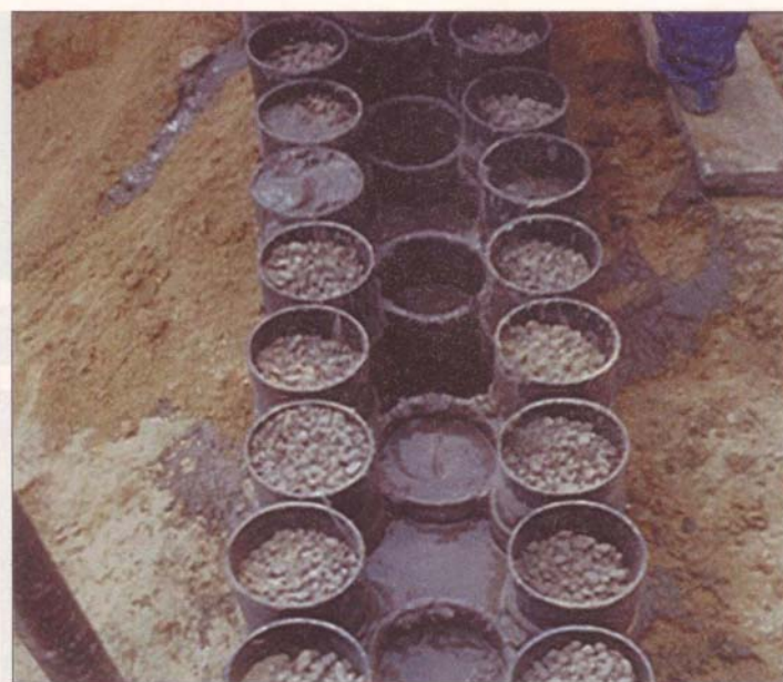
Figure 12.4 Photograph showing a prototype vertical barrier system using HDPE pipes (after Gallagher et al. 2000)
