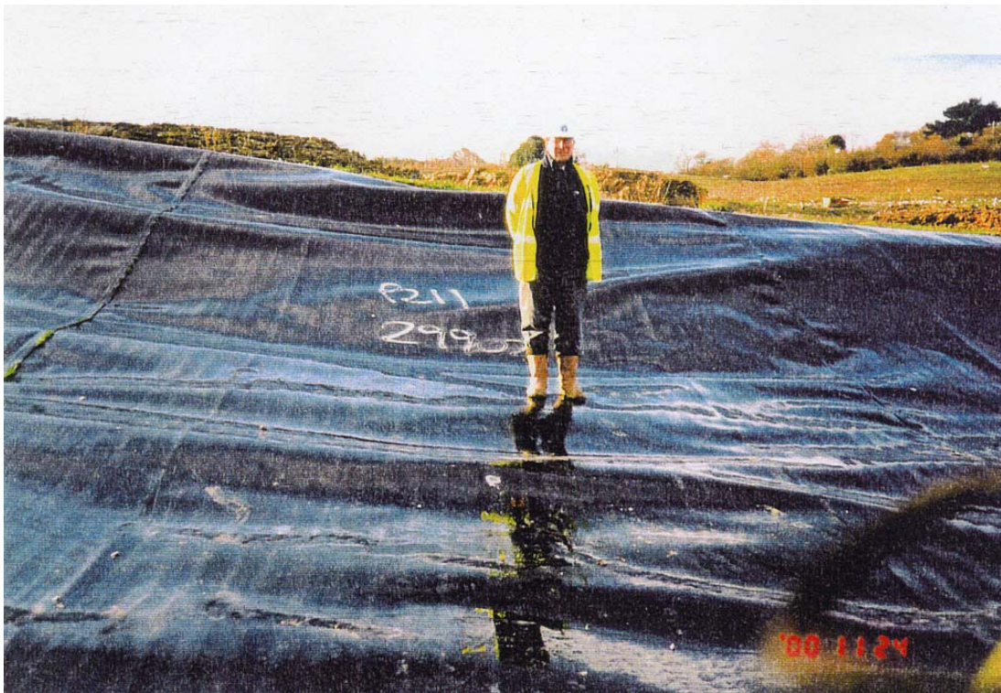
Figure 4.11 Distress of geomembrane following failure of the southern bund
