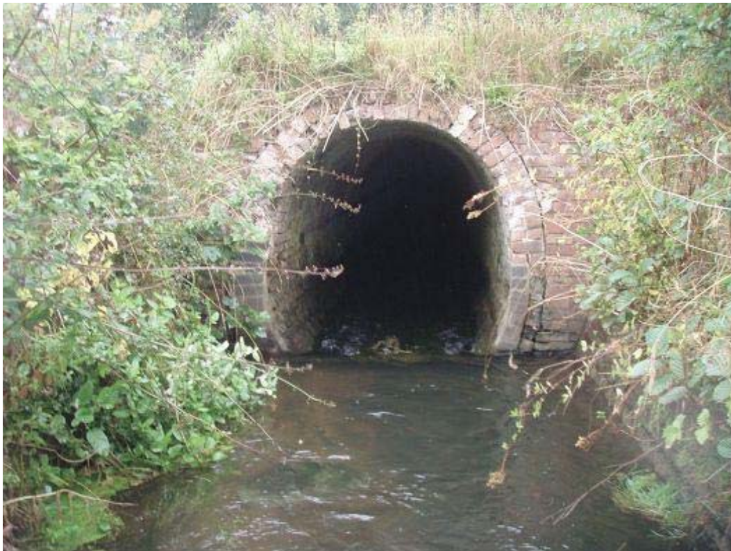
Figure 1.3. Head of 720 metre culvert taking 50% of the Glaven's flow on the Bayfield Estate (photo with thanks to Tim Jacklin, Wild Trout Trust).
