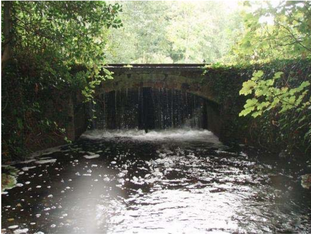
Figure 1.2. Impassable spillway at downstream end of Bayfield Estate lake (photo with thanks to Tim Jacklin, Wild Trout Trust).
