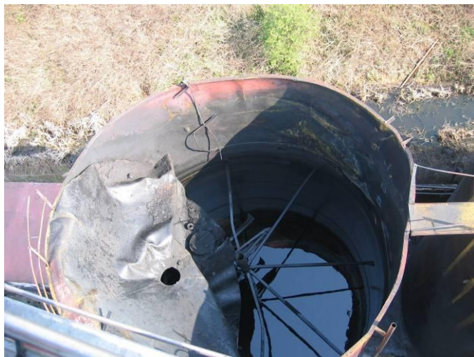
Figure 4 - Tank 4 after explosion
