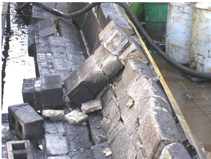
Figure 2 - Collapsed bund wall
