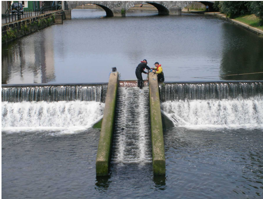
Figure 11: Installing equipment on Haverfordwest Town Weir fish pass (1,500 mm wide Larinier fish pass)
