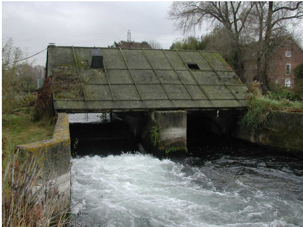
Figure 3.5: A covered resistivity weir lit by fluorescent tubes, River Test
