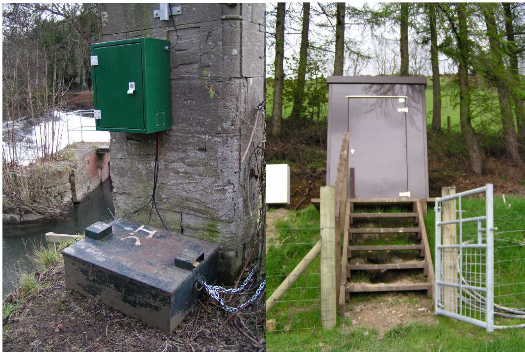
Figure 3.1: Examples of housing. The metal box houses a bank of three batteries powering lighting and recording equipment in the green wall mounted cabinet. In the second photograph is a GRP hut installed on a concrete base.
