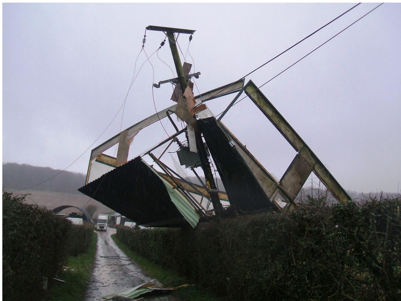
Farms structure blown on to electricity pylon and lines
