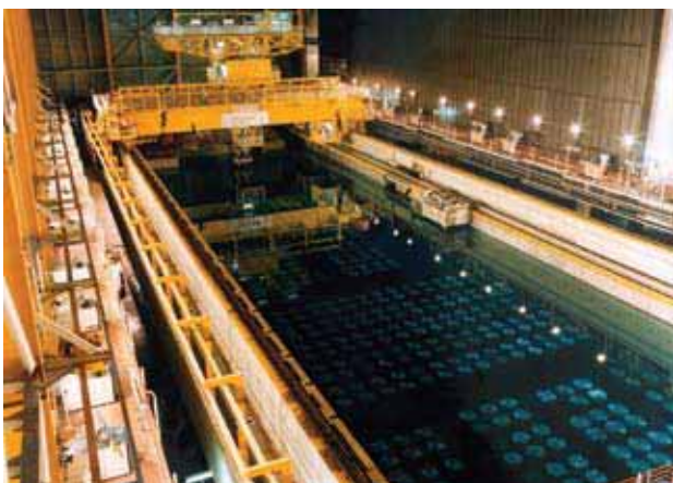
Storage Pond in (THORP) Thermal Oxide Reprocessing Plant Receipt and Storage at Sellafield
