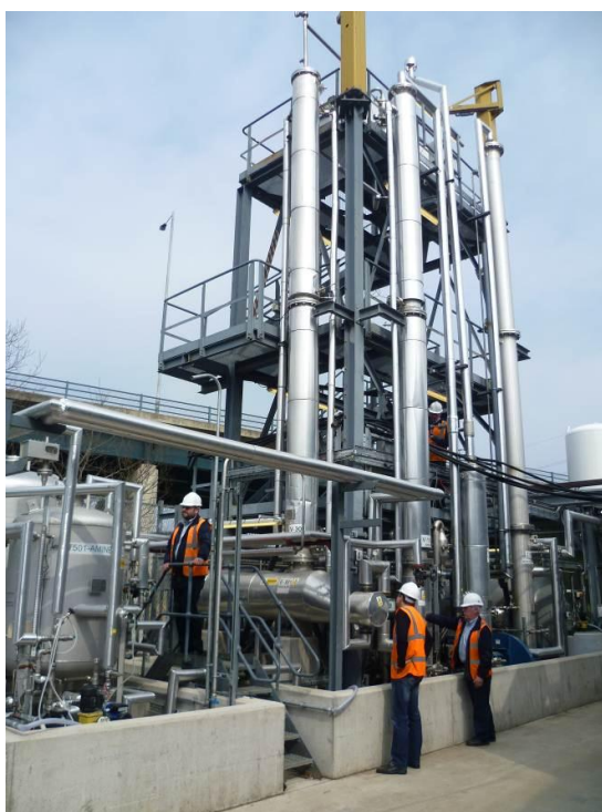
Figure 2: CCS Research Facilities – The PACT Carbon Capture Plant in Sheffield
