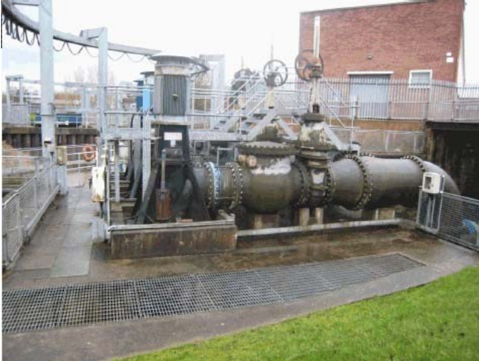
Figure A2.6 Crossens external Sluice pumps
