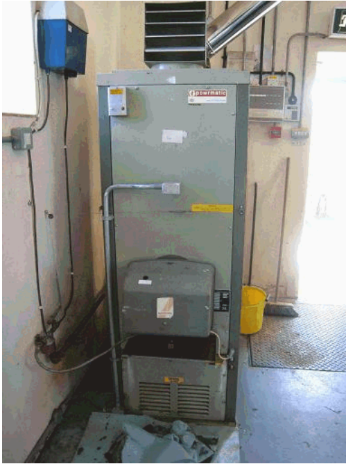
Figure 7.6 The oil fuelled fan heater in the main pump building at West Sedgemoor
