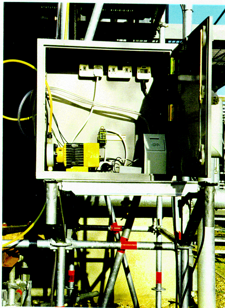
Plate 4. Control cabinet showing pump, timer, temperature logger and gasflow meter
