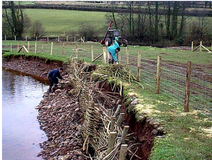
Figure 49 Staked woven willow panels used to reinstated bank on this badly eroded river bend. The fencing will prevent livestock incursion
