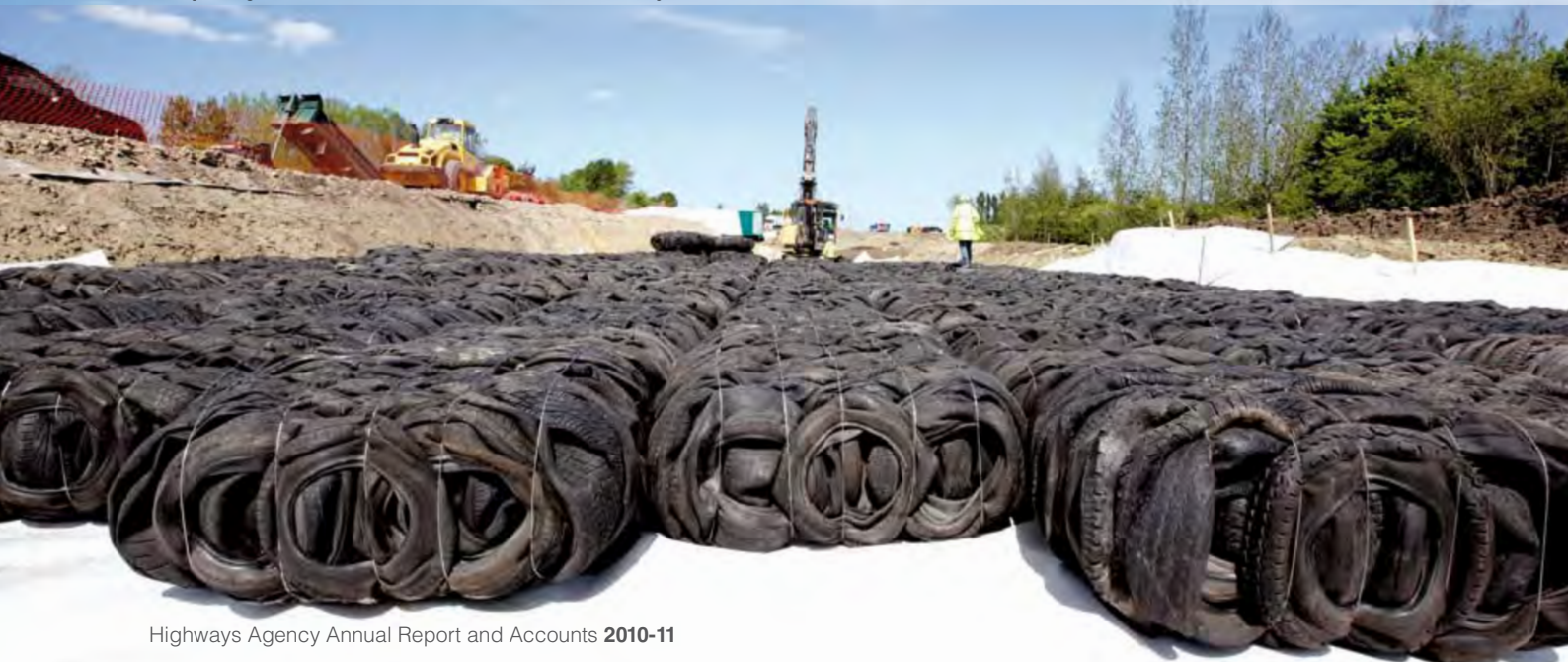
Recycling waste material – innovative use of tyre bales in the A421 scheme
