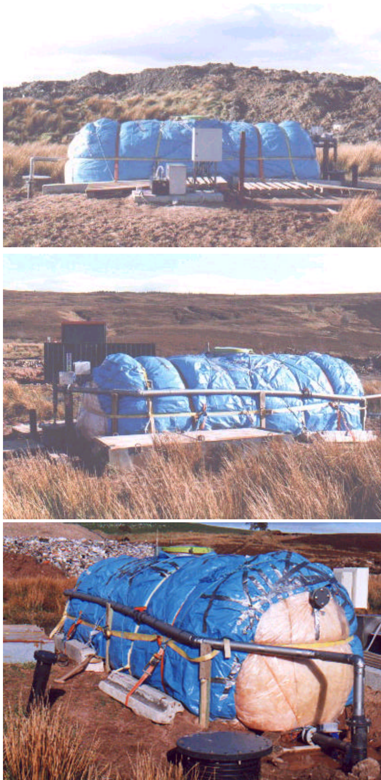
Figure 4.2 The aeration tank.
