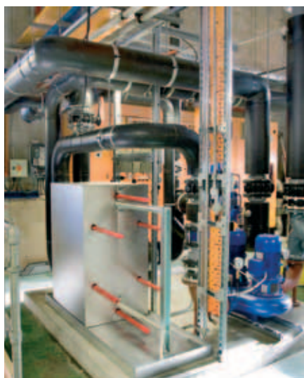
The Sea Water Cooling Systems Heat exchanger at the National Oceanography Centre, Southampton.
