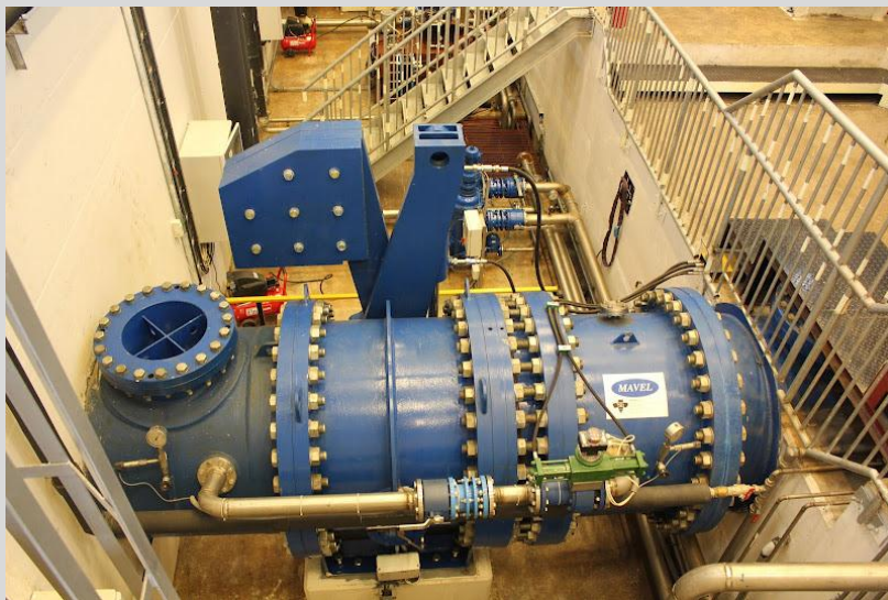
Bugoye Pump House. Photo credit: DFID Private Sector Department
