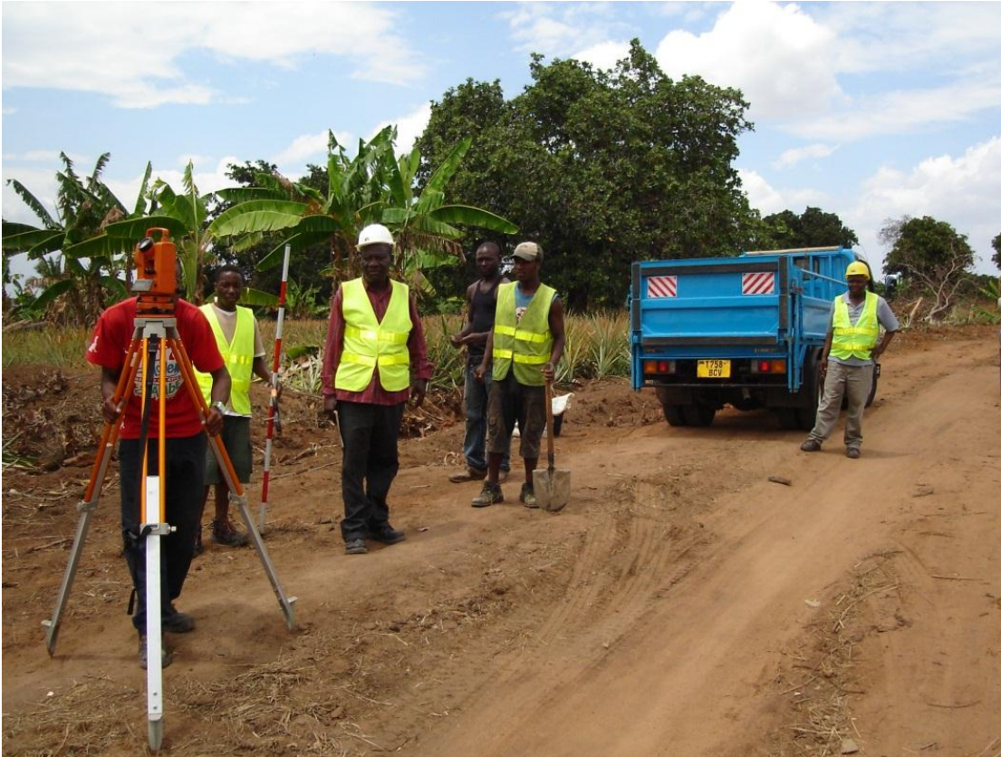
Road improvement works in Bagomoyo, Tanzania following AFCAP guidance. Photo credit: Crown Agents
