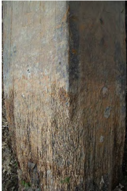
Figure 2.19 Gribble attack on Timber pile at the sediment line (courtesy of HR Wallingford)
