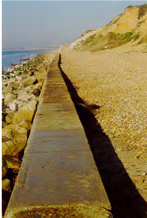
Figure 3.7 Repaired wall showing failed realignment. Rock armour has been added at the toe (courtesy A P Bradbury)
