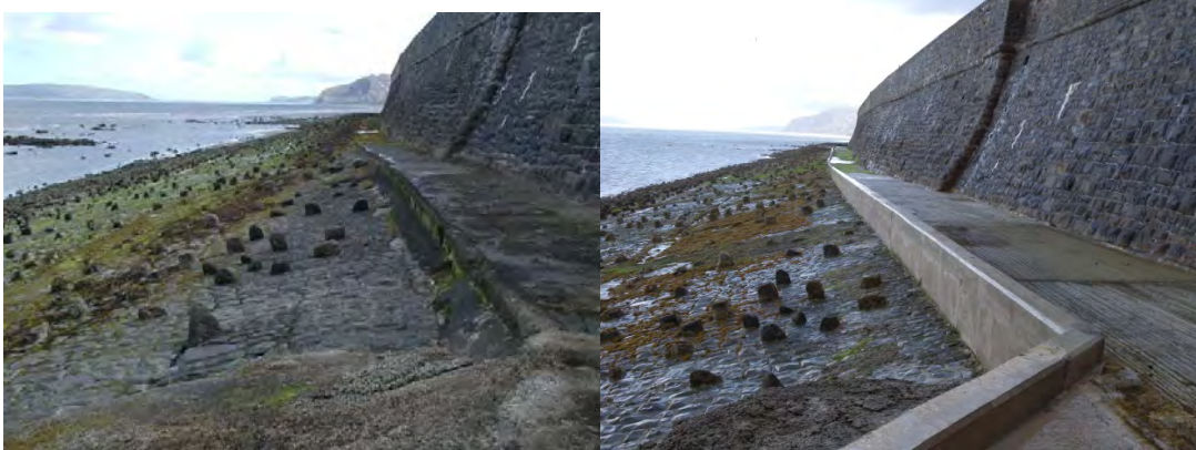
Figure 4.7 Improvement of access by construction of concrete roadway suitable for plant access (courtesy Alan Williams)
