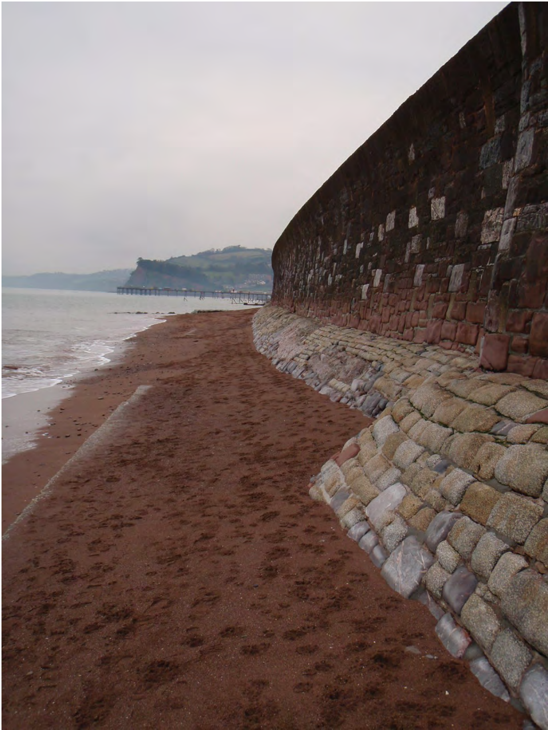
Figure C7.6 Partial foundation strengthening – Sprey Point to Teignmouth (note only outer edge of single step visible at the time photo was taken)
