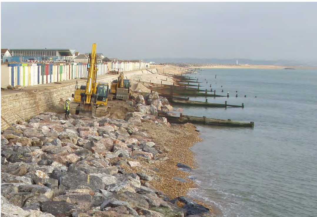
Figure 4.6 Improvement of access by construction of rock toe with wide crest berm suitable for plant access (courtesy New Forest District Council)
