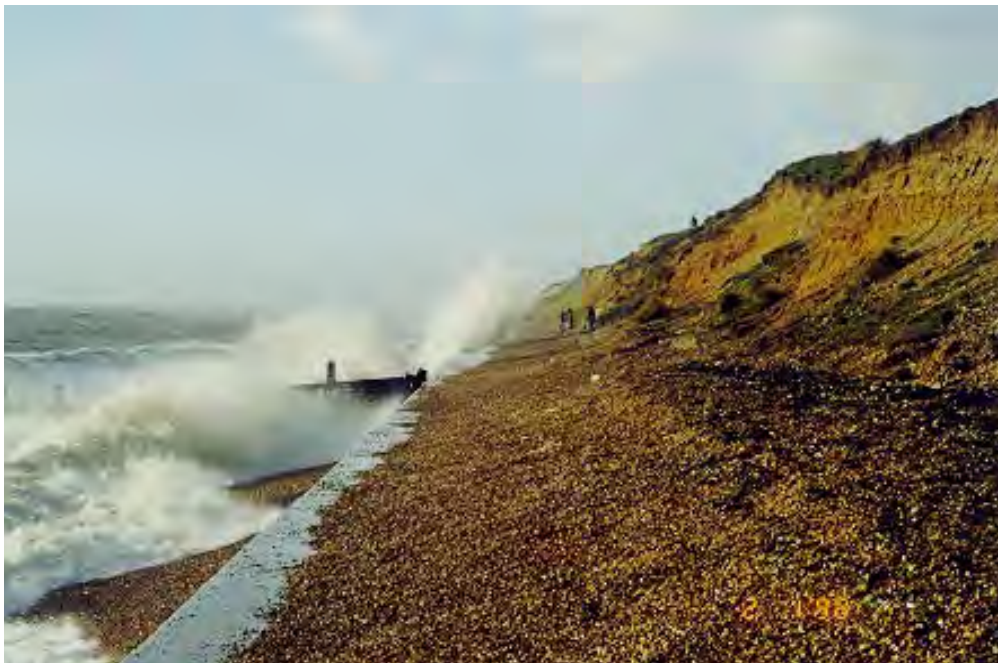
Figure 3.6 Frequent overtopping causes build-up of pressure on landward side of seawall (courtesy A P Bradbury)
