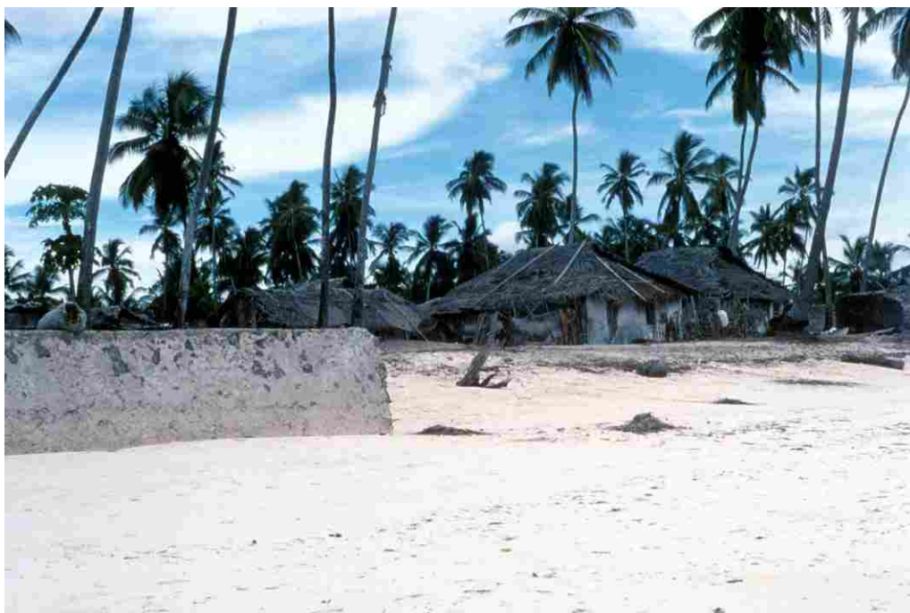
Figure A.18 Erosion at downdrift end of seawall, Zanzibar
