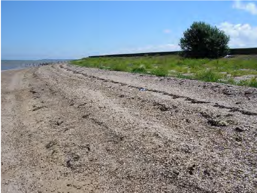
Figure 4.17 Vegetation growth on a revetment (courtesy ENBE)
