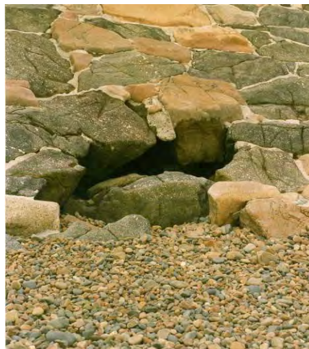
Figure 4.20 Dislodged masonry blocks from revetment toe (courtesy HR Wallingford)
