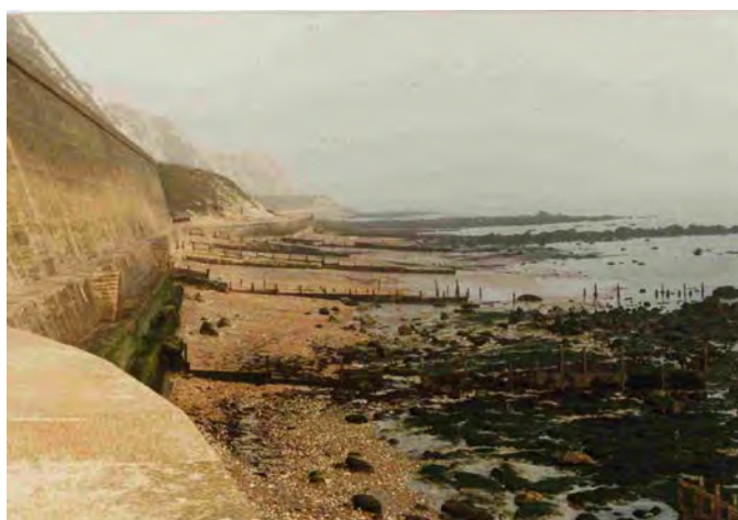
Figure 3.26 An extreme example of beach depletion, foreshore erosion and down-cutting – note the level of the base of the access steps in relation to the level of the beach (courtesy HR Wallingford)
