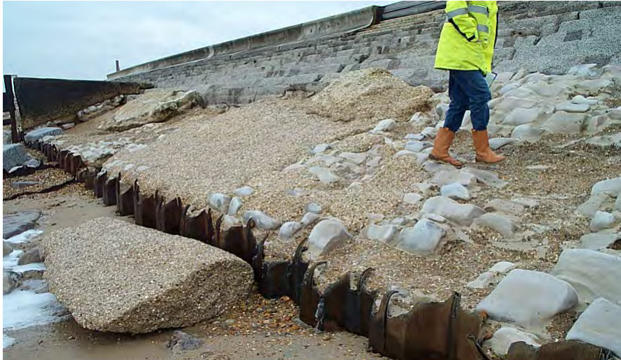
Figure 4.4 Typical damage to tops of steel interlocking piles (courtesy AP Bradbury)
