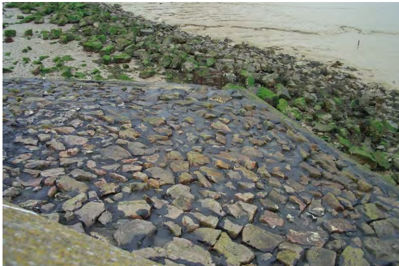
Figure 2.18 Asphalt grouted stone revetment in the Thames Estuary (courtesy HR Wallingford)
