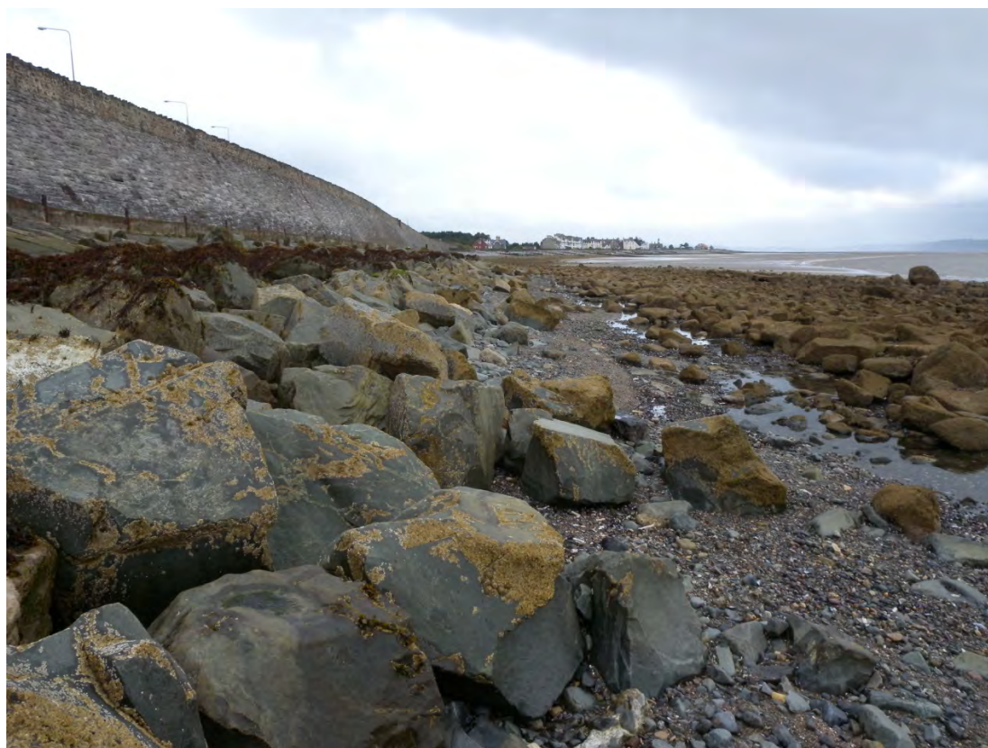
Figure 4.15 Armour displaced from a rock toe, Llanfairfechan, North Wales (courtesy Alan Williams)
