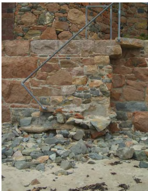
Figure 3.30 Beach lowering at access steps (courtesy HR Wallingford)
