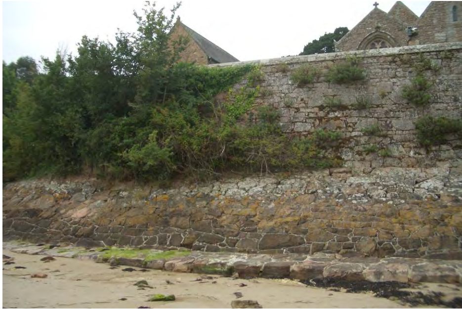
Figure 4.17 Vegetation colonising joints in a masonry coastal defence (courtesy HR Wallingford)
