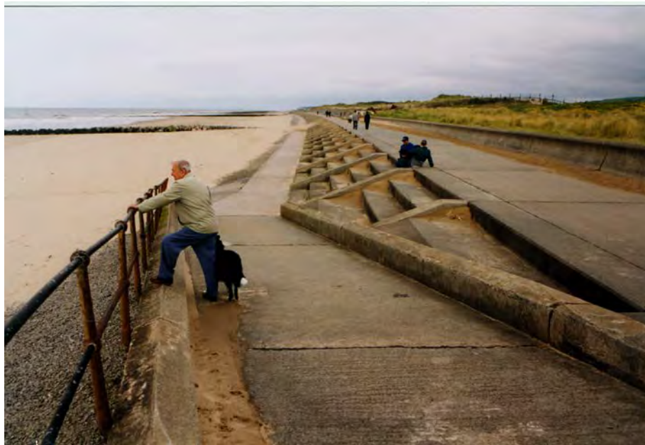
Figure C11.2 Sloping asphalt apron and rock groynes in front of steeped concrete seawall
