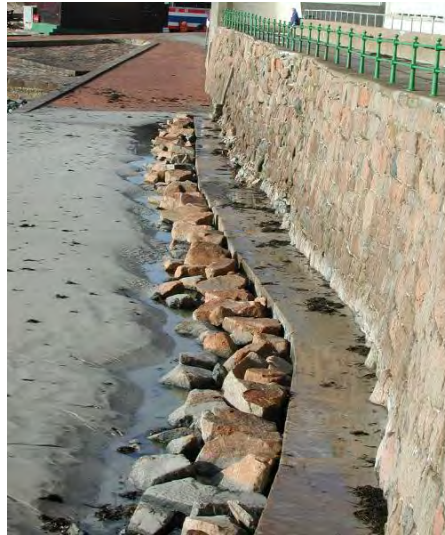
Figure 2.6 Rock infill of scour trough, Le Dicq, Jersey (courtesy HR Wallingford)
