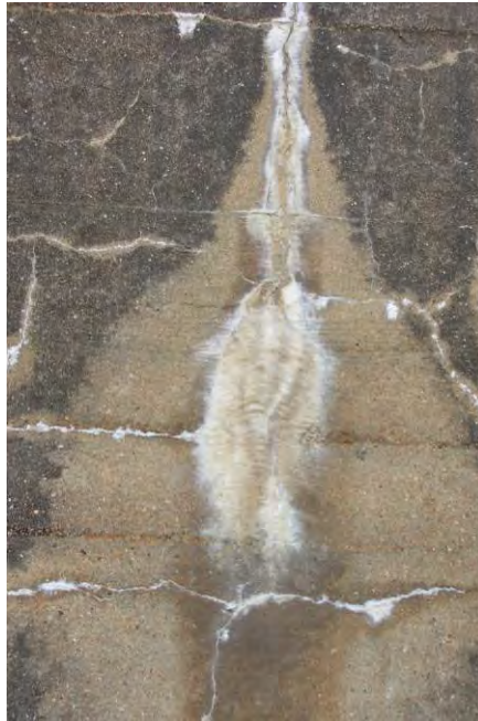
Figure 2.16 Surface salt deposits and associated cracking from alkali–silica reaction in concrete (courtesy of HR Wallingford)
