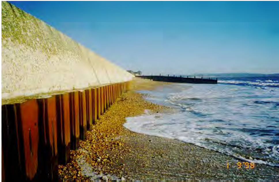
Figure 3.5 Exposure of interlocking steel piled toe arising from beach lowering (courtesy A P Bradbury)
