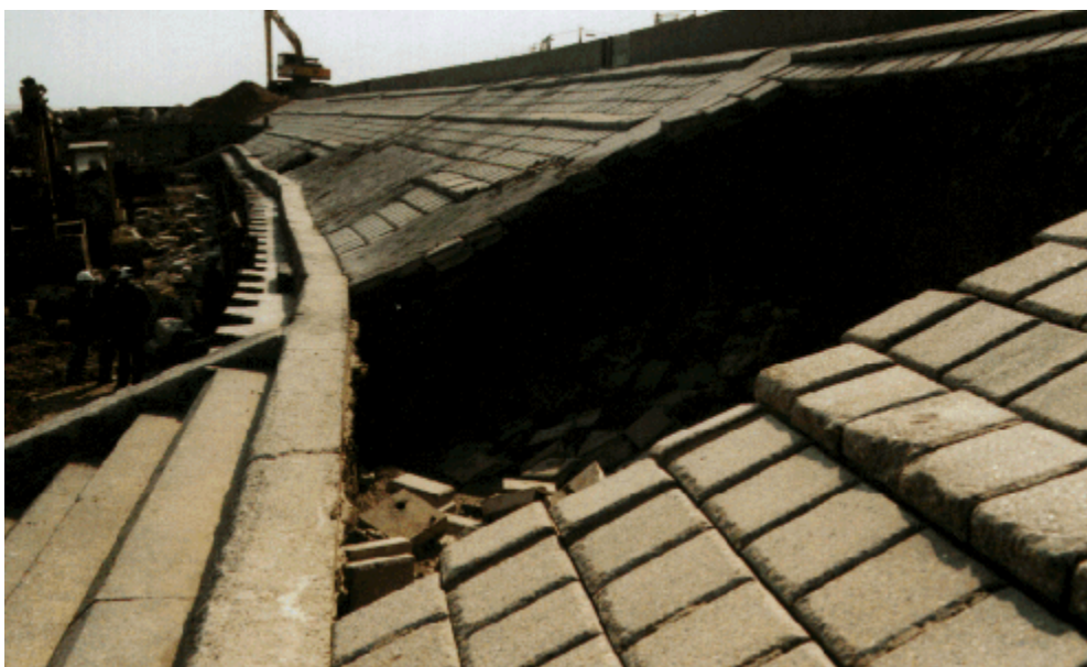
Figure 4.21 Washout and collapse of block revetment following block removal (courtesy Canterbury City Council)
