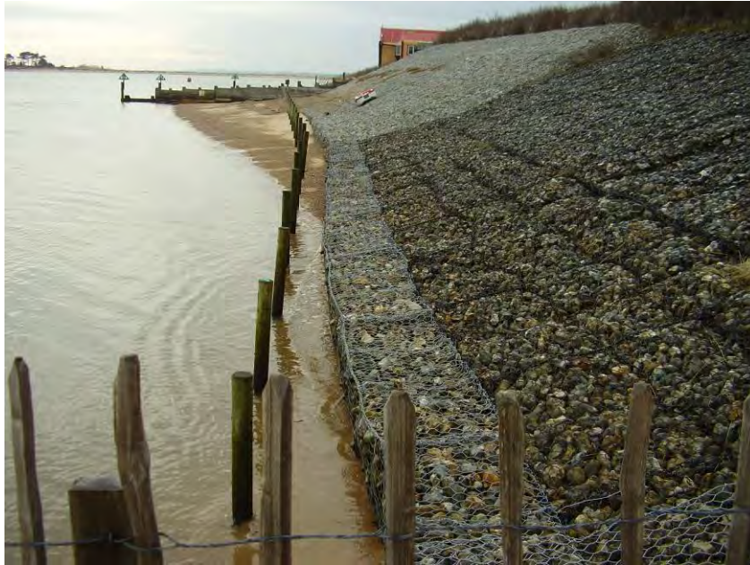
Figure 2.5 Gabion baskets of rock (courtesy HR Wallingford)
