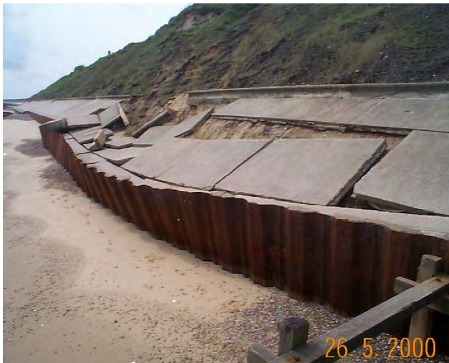
Figure C2.5 Rotation of the toe piling (photograph taken after the 1999 failure)
