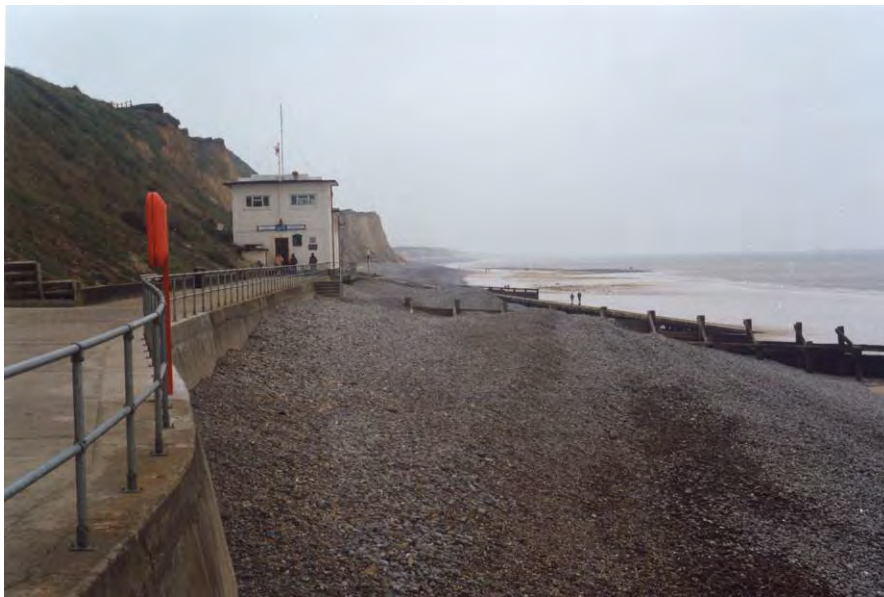
Figure A.17 Accumulation of shingle at updrift end of seawall, Sheringham, Norfolk
