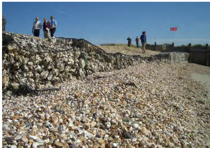
Figure 4.16 Weathered gabions at East Head, Chichester Harbour, West Sussex (courtesy HR Wallingford)
