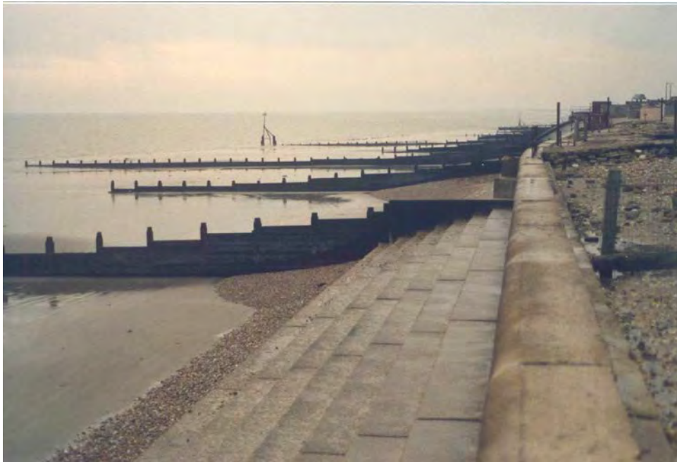
Figure C17.1 Low beach levels in front of stepped concrete wall, 1988
