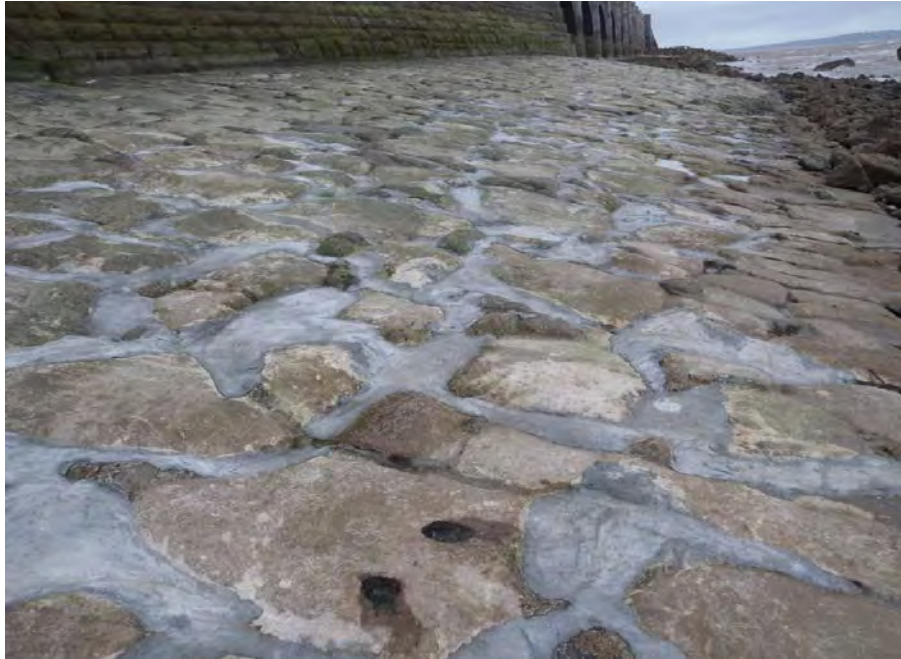
Figure 4.19 Prior to and following maintenance of grouted masonry toe (courtesy Alan Williams)
