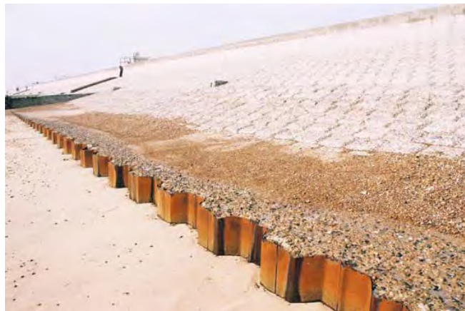
Figure C8.5 Exposed toe piling at Environment Agency frontage, 2003
