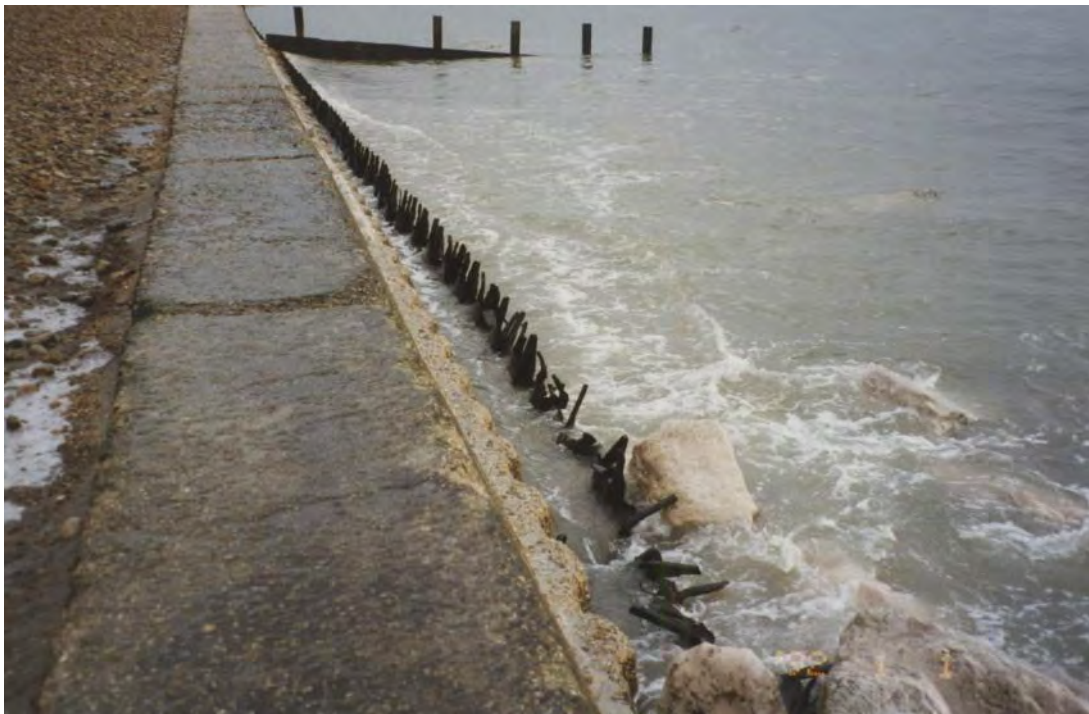
Figure 4.24 Damaged interlocking steel piles requiring maintenance to make site safe (courtesy A P Bradbury)
