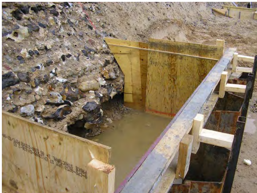
Figure C3.7 Shuttering for concrete thrust block (apron) – old flint wall section (note water ingress and exposure of the toe of the existing wall)
