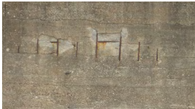
Figure 3.29 Exposed reinforcing mesh due to steel oxidation and resultant cracking and flaking of concrete cover layer (courtesy HR Wallingford)
