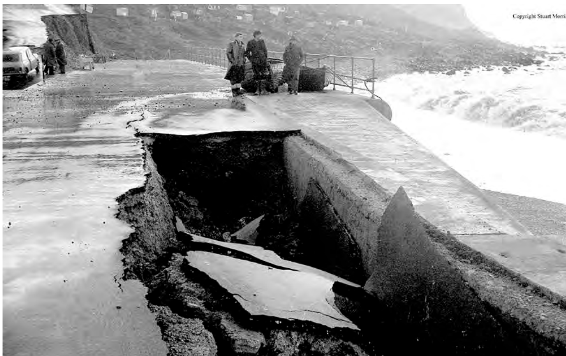
Figure 4.12 Typical collapse of promenade decking following undermining of backfilled mass concrete wall and washout of fine core (Chesil Cove 1962) © Stuart Morris
