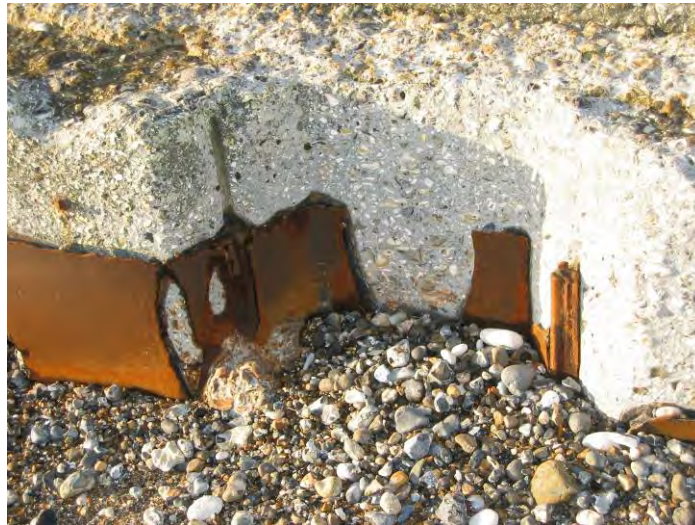
Figure 4.23 Complete loss of section of sheet piles in an area exposed to sediment movement
