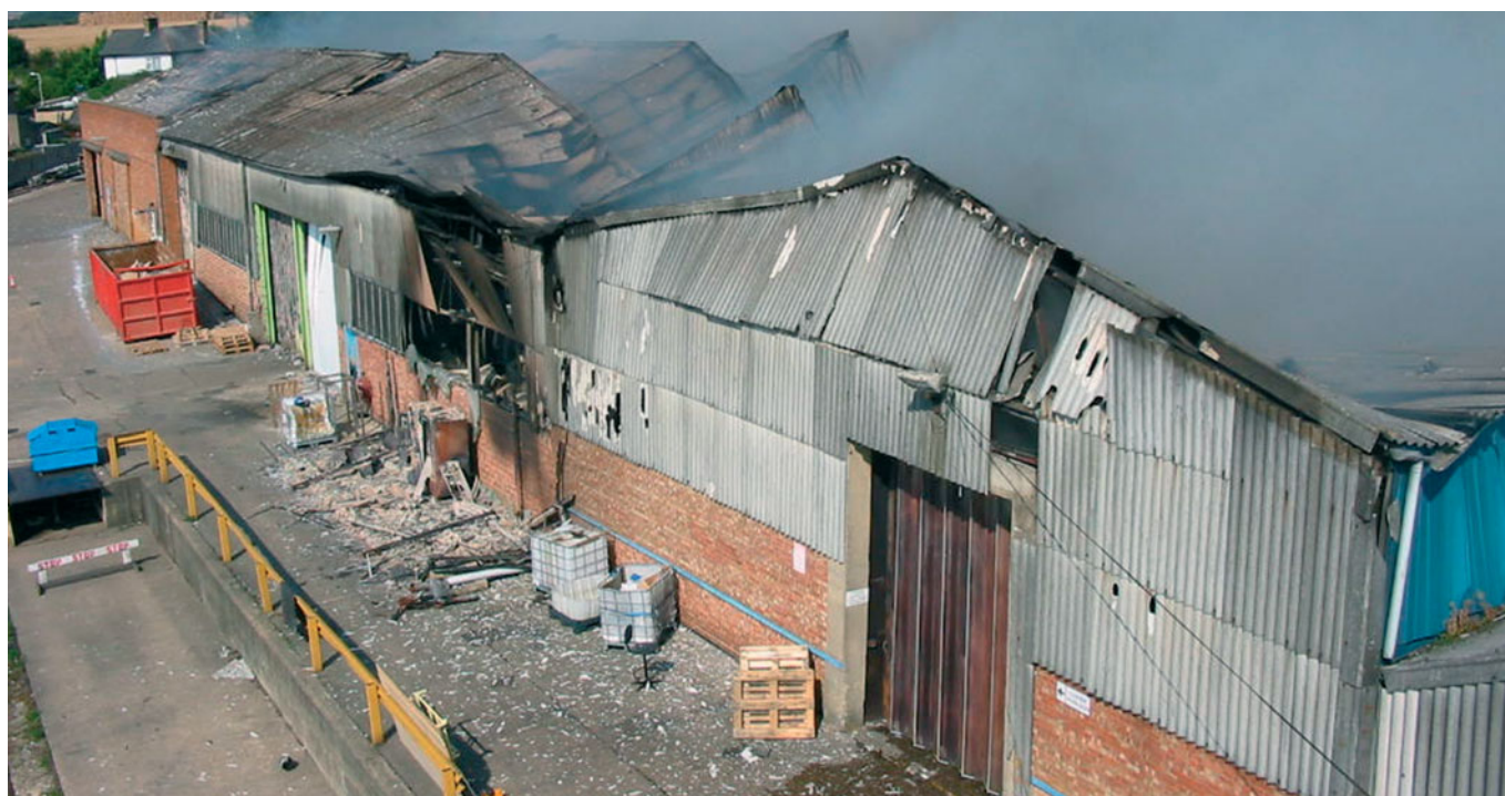
Figure 1: Fire at a commercial property involving asbestos. © HPA, 2003
