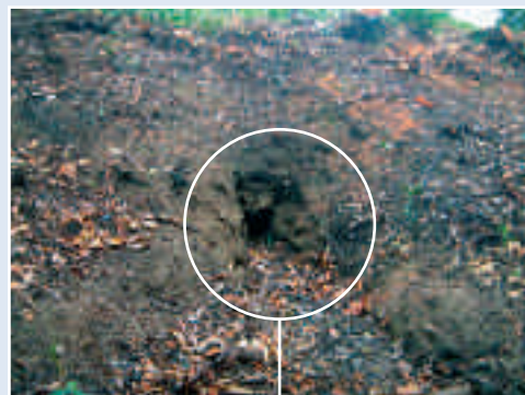
Erosion hole at toe of dam
