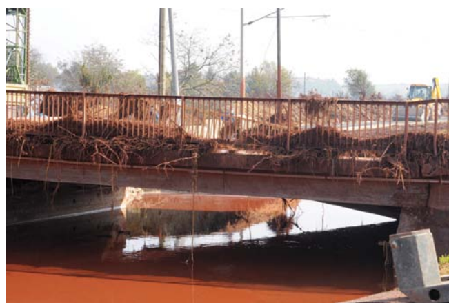
Figure 2: After-effects of the Ajka alumina sludge spill at the Ajkai Timföldgyár alumina plant in Veszprém County in Western Hungary
