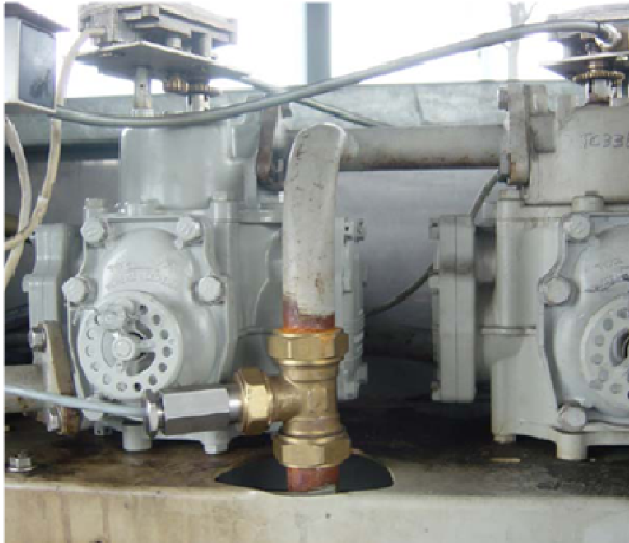
Figure 26 Typical installation of temperature sensor
