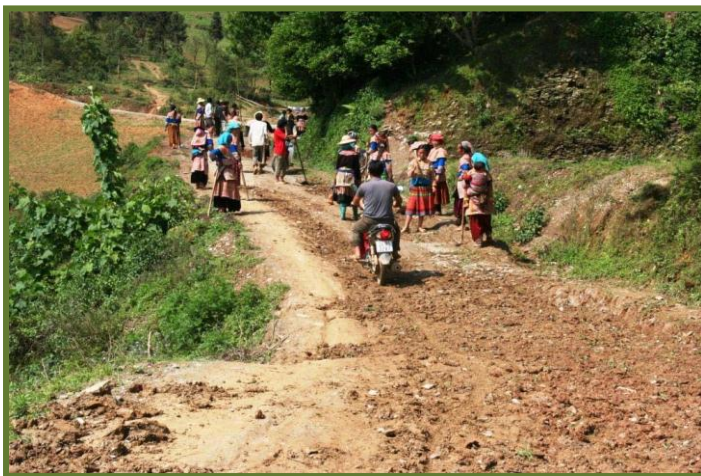
Ethnic minority women engaged in maintenance work on rural roads under the Rural Transport Programme (RT3) in Lao Cai province. RT3 will help improve access to 3,000 communes and lift 320,000 people out of poverty (Source: Phan Manh Tuan, RT3 Consultant)
