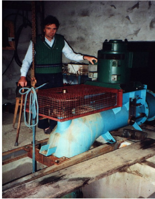
Figure 5.6 7kW propeller turbine and generator, on 3m head, Evans Engineering Ltd
