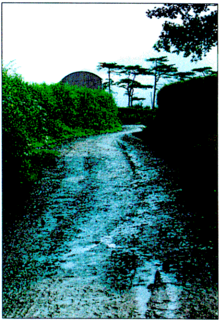
Sediment and organic waste on green lanes – commonly transmitted to river during high rainfall
